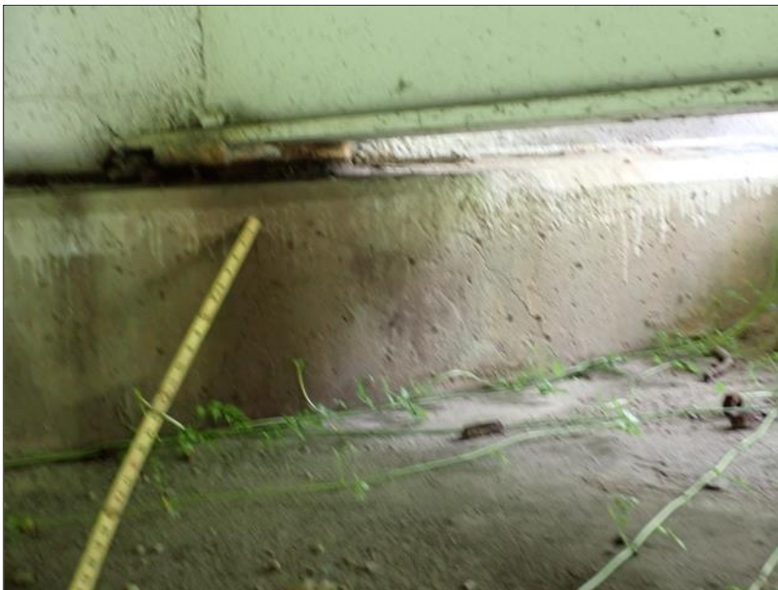
End Bent 2 Cap 1: 2 FEET HIGH X 1/32 INCH WIDE DIAGONAL CRACK UNDER BEAM 4.
