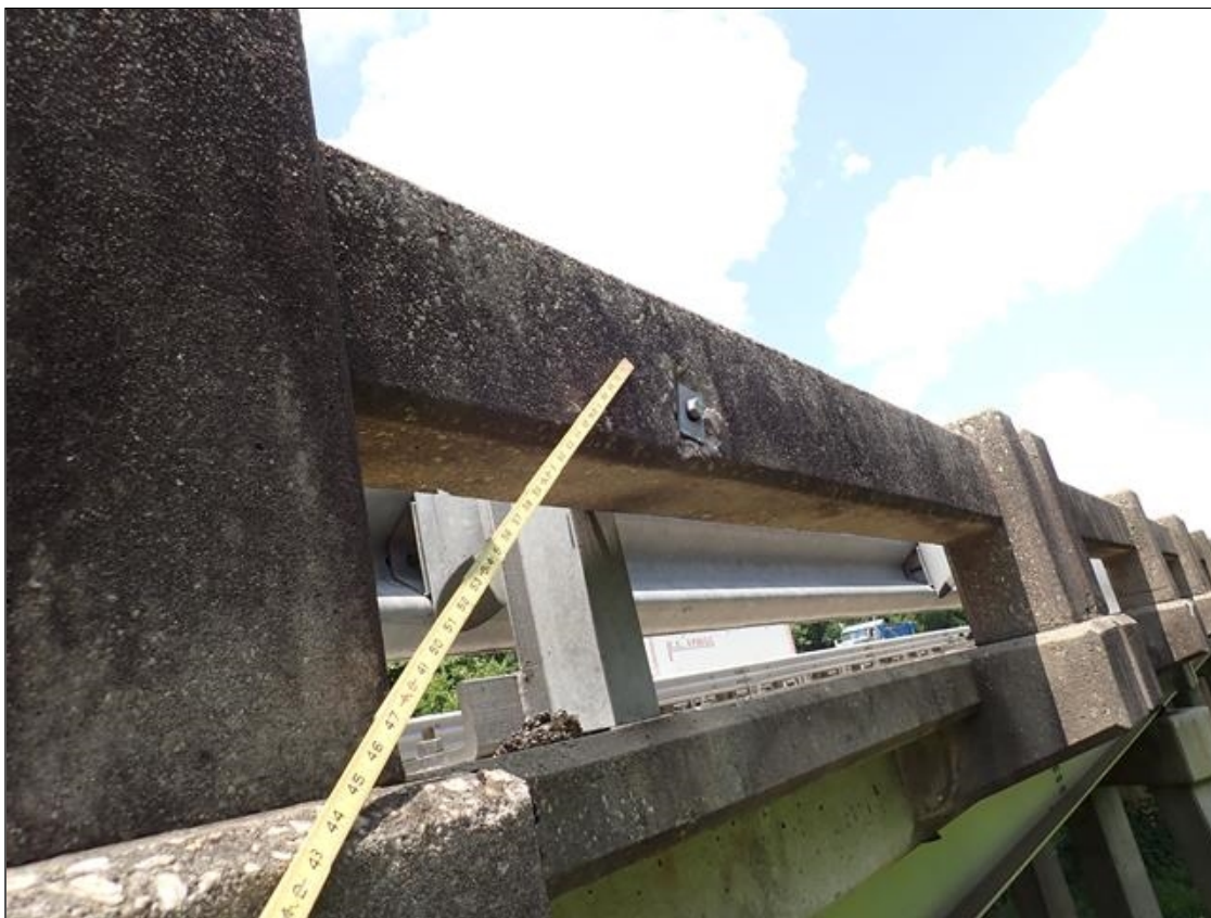
Span 1 Right Bridge Rail: UP TO 6 INCH DIAMETER X 1.5 INCH DEEP SPALL IN EXTERIOR FACE AT ANCHOR BOLT CONNECTION. TYPICAL AT SEVERAL CONNECTIONS.
