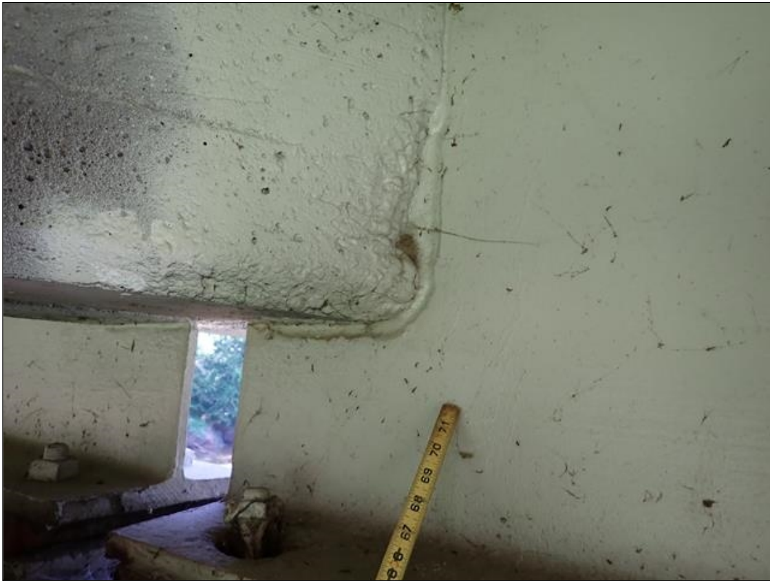
Span 2 Beam 4: (PAR) at bent 2, web adjacent to end diaphragm, painted over section loss (1/2 inch average remaining x 12 inch x 9 inch)
