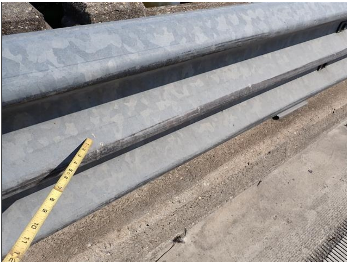
Span 3 Left Retrofit Bridge Rail: along the length of the rail, impact scrapes at random
