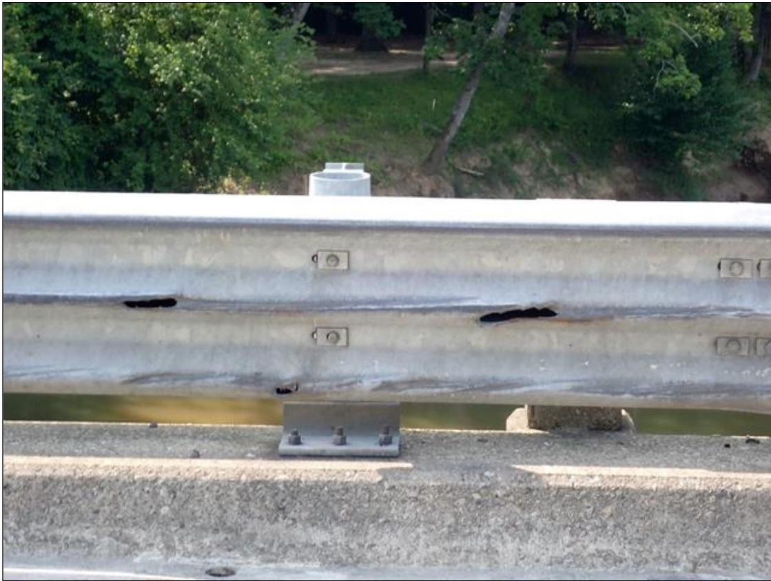
Span 4 Right Retrofit Bridge Rail: (PAR) IMPACT DAMAGE WITH SCRAPE MARKS AND THROUGH HOLES UP TO 4 INCH X 2 INCH IN RETROFIT RAIL AT SCATTERED LOCATIONS
