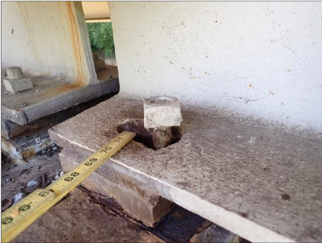
Span 4 Far Bearing 1: RIGHT ANCHOR BOLT IS MISSING; LEFT ANCHOR BOLT, PAINTED OVER SECTION LOSS (50 PERCENT REMAINING); WELDED REPAIR WITH NEW ANCHOR BOLTS.
