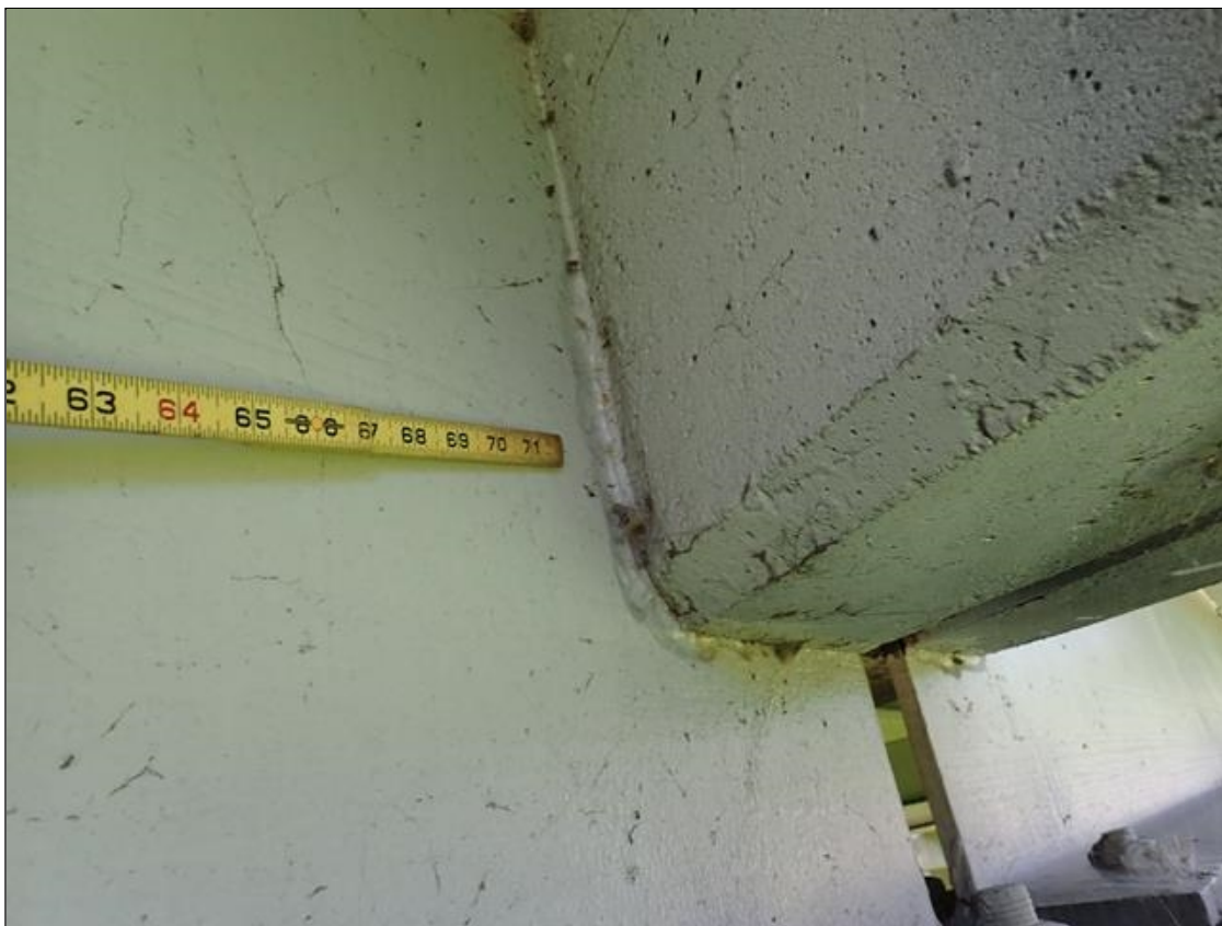
Span 3 Beam 1: at bent 2, web adjacent to end diaphragm, painted over section loss (1/2 inch average remaining x 1 inch x 8 inch)
