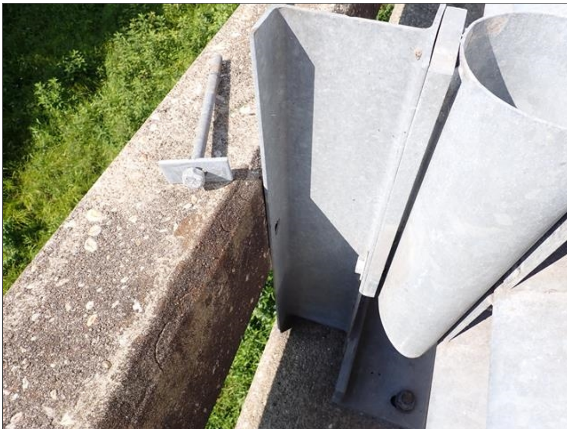
Span 2 Right Retrofit Bridge Rail: (PAR) BOLT HAS DETACHED FROM CONCRETE OUTER RAIL 10 FEET FROM BENT 1 LEAVING METAL INNER RAIL FREE
