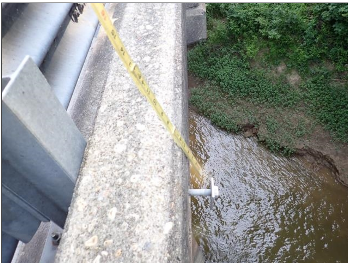
Span 6 Right Retrofit Bridge Rail: (PAR) ADJACENT TO POSTS 5 AND 8, 2 BOLTS DISCONNECTED AND PROTRUDING ON THE OUTSIDE OF RAIL
