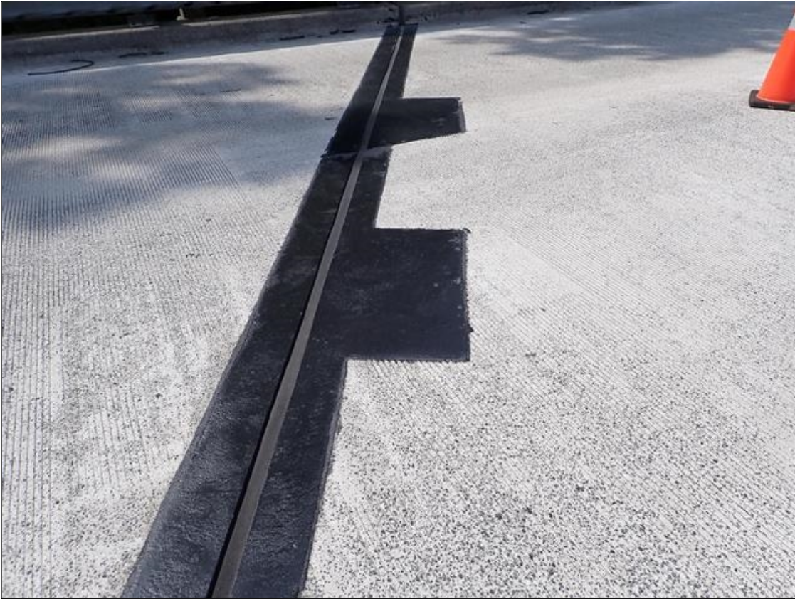
Span 7 Bent 6 Joint: 2025 NEW REPAIR (UP TO 37 INCH X 24 INCH), PREVIOUSLY NOTED AS: IN RIGHT AND LEFT LANES (2) AREAS OF MISSING HEADER AND JOINT MATERIAL UP TO 2 FEET X 8 INCHES X FULL DEPTH
