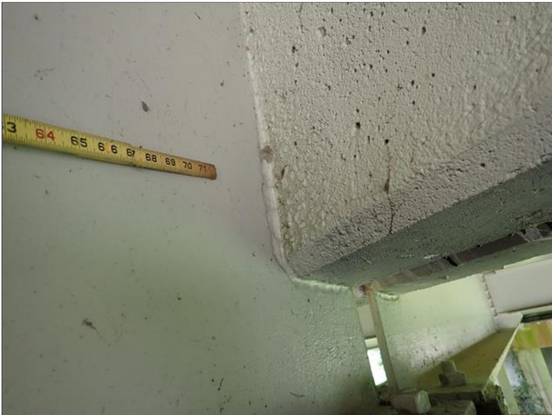
Span 6 Beam 3: (PAR) at bent 6, web adjacent to end diaphragm, painted over section loss (3/8 inch average remaining x 8 inch x 8 inch) with corrosion reactivating
