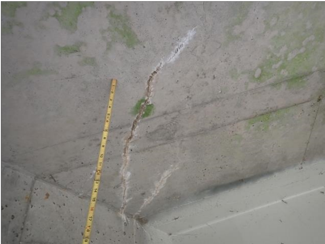
Span 6 Deck: UP TO 0.02 INCH WIDE RANDOM CRACKING SOME WITH EFFLORESCENCE IN DECK UNDERSIDE, SCATTERED THROUGHOUT.
