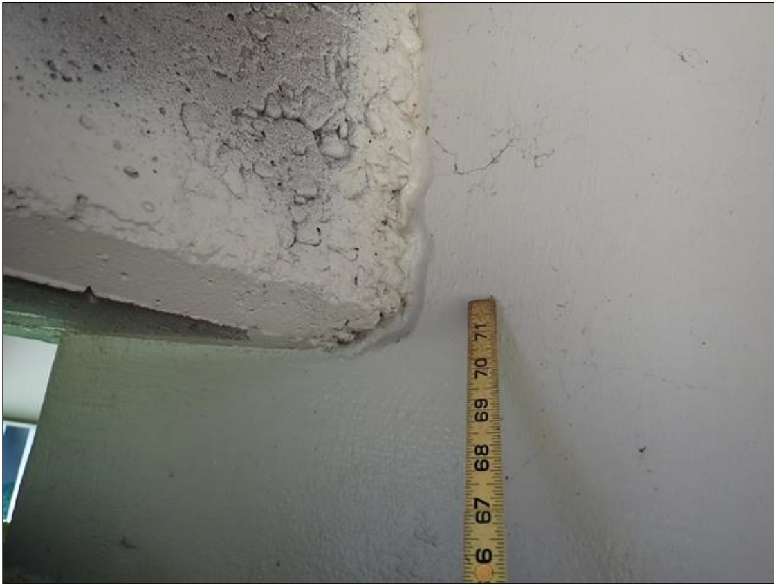
Span 4 Beam 2: (PAR) at bent 3, web adjacent to end diaphragm, painted over section loss (3/8 inch average remaining x 10 inch x 1 inch)
