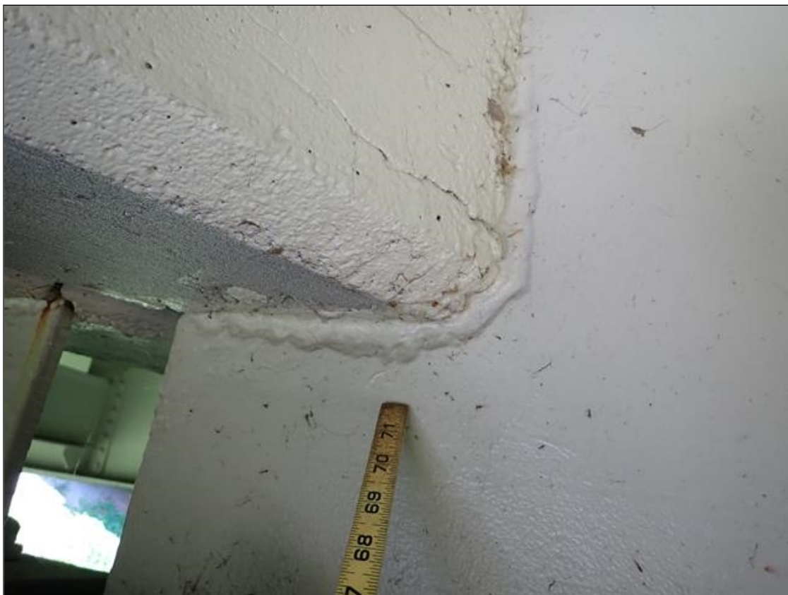
Span 3 Beam 3: (PAR) at bent 2, web adjacent to end diaphragm, painted over section loss (3/8 inch average remaining x 10 inch x 7 inch)
