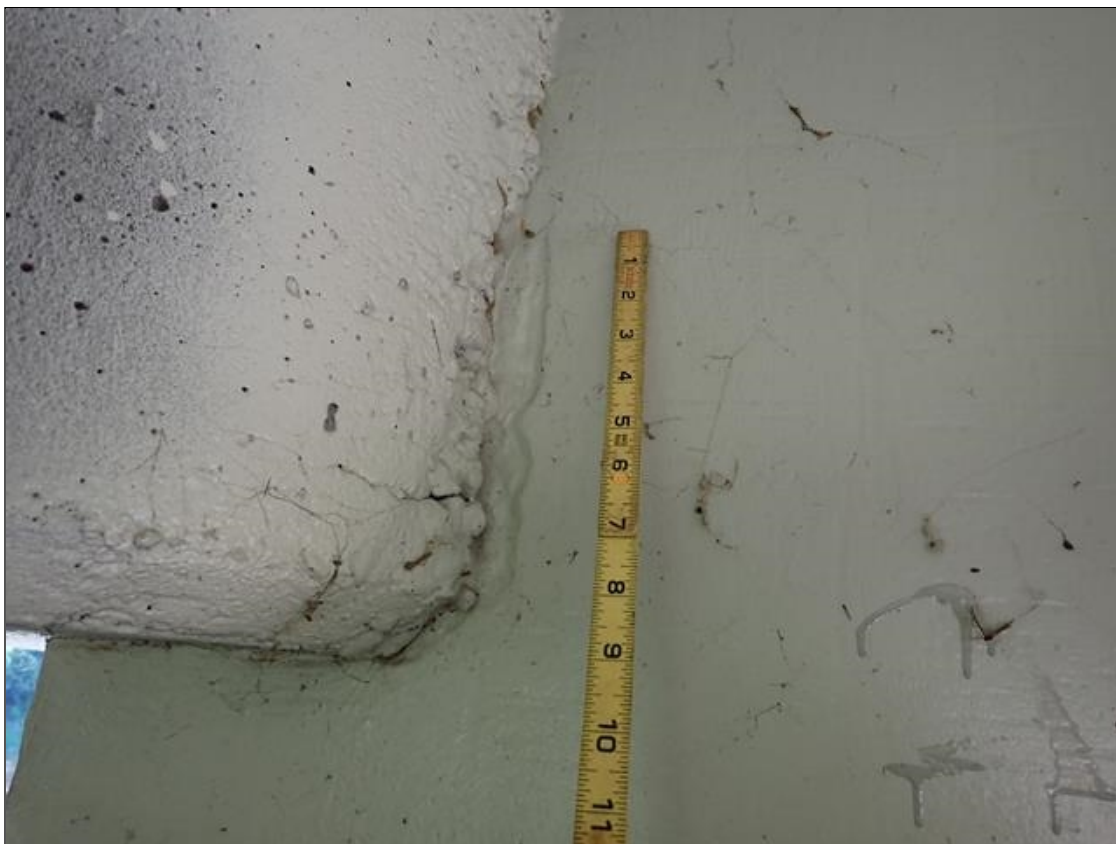
Span 1 Beam 4 : at bent 1, web adjacent to end diaphragm, painted over section loss (9/16 inch average remaining x 1.5 inch x 8 inch)
