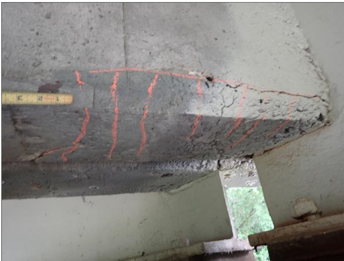
Span 5 Deck: bay 3 end diaphragm over bent 5, delamination (20 inch x 10 inch) with cracks (up to 1/16 inch)
