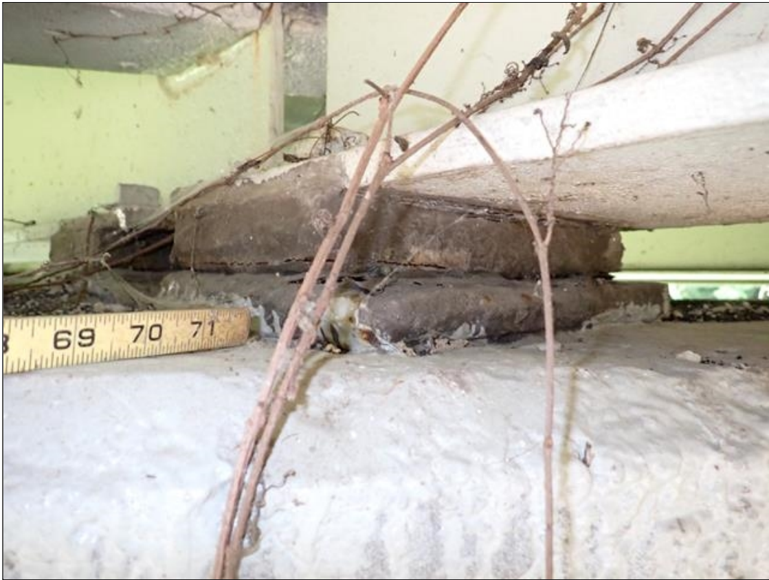
Span 7 Far Bearing 2: painted over section loss (approximately 85 percent remaining)
