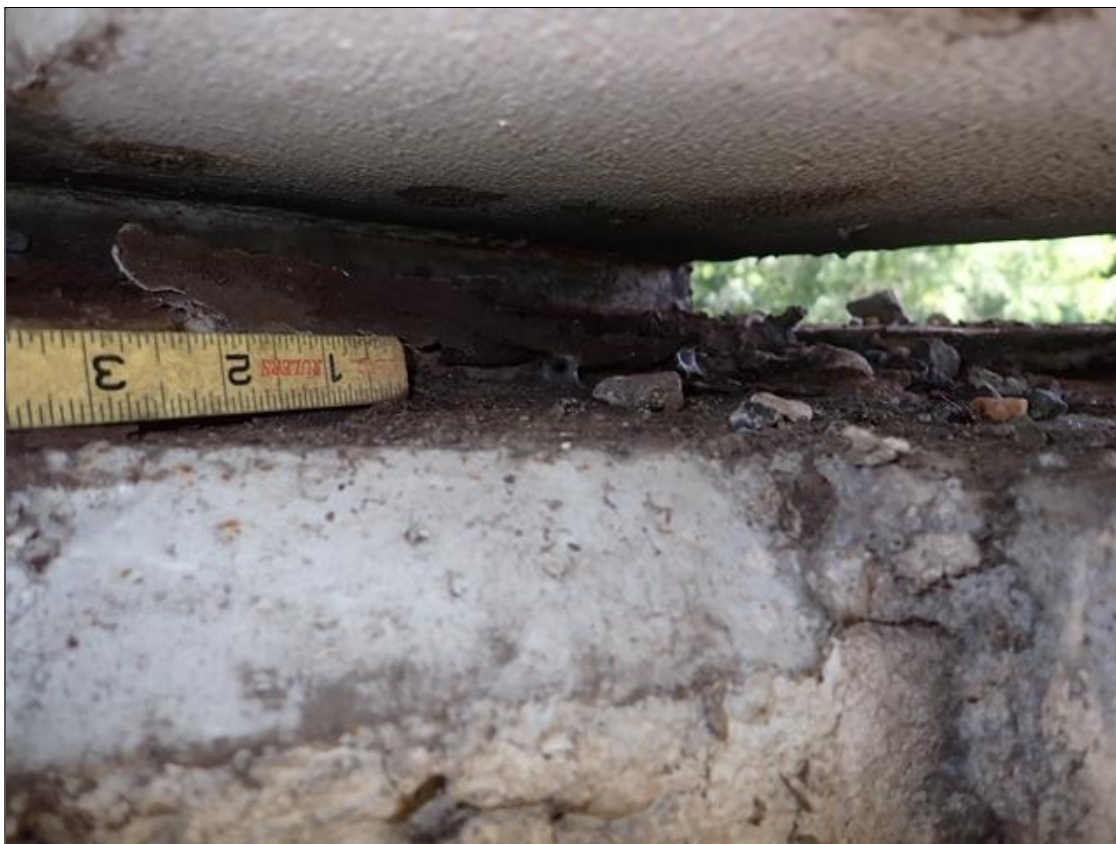
Span 4 Far Bearing 4: corrosion with section loss (approximately 80 percent remaining)
