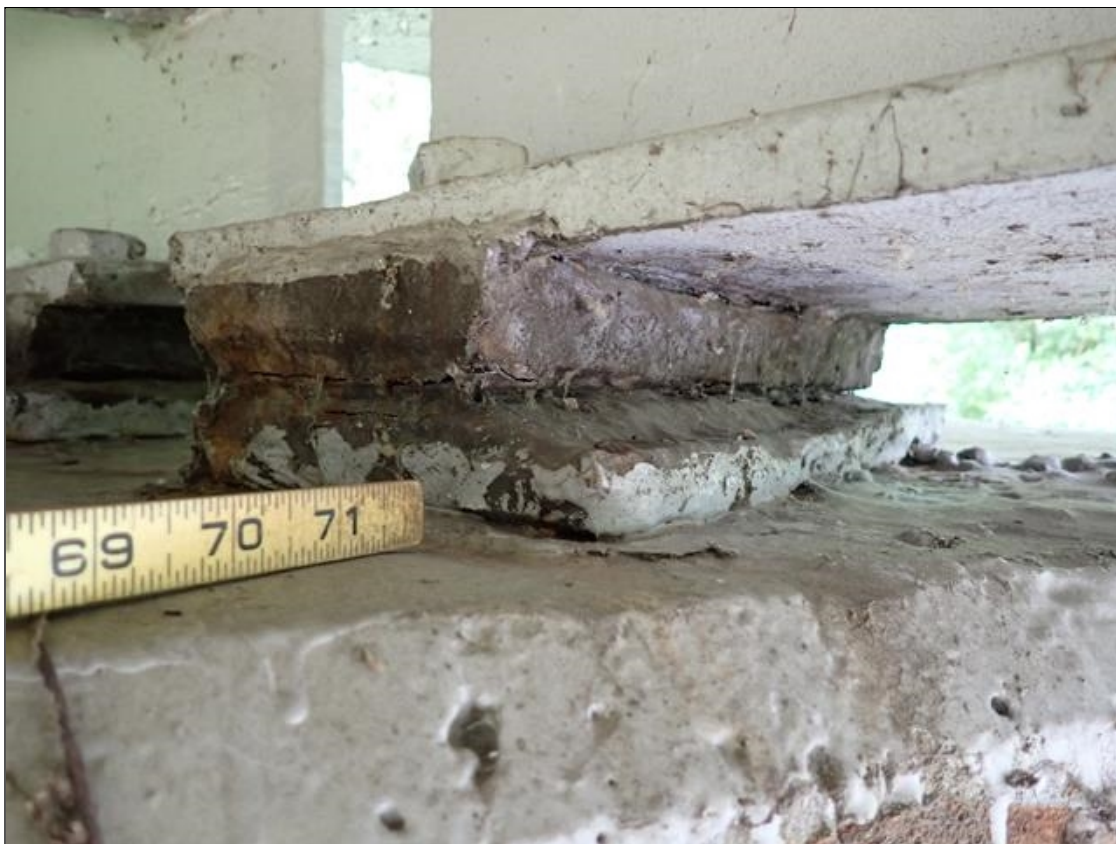
Span 7 Far Bearing 4: painted over section loss (approximately 80 percent remaining)
