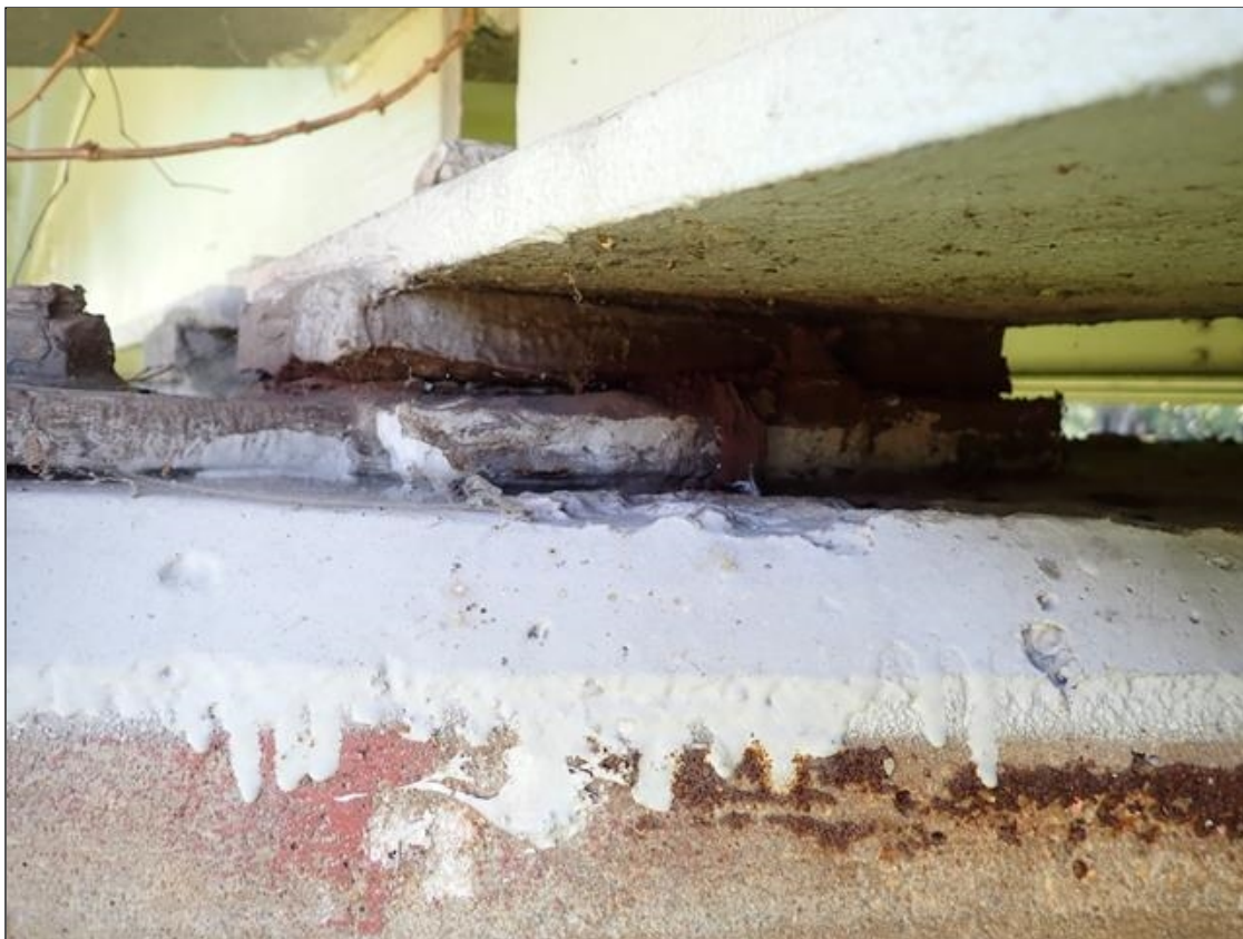
Span 1 Far Bearing 1: painted over section loss (approximately 80 percent remaining)
