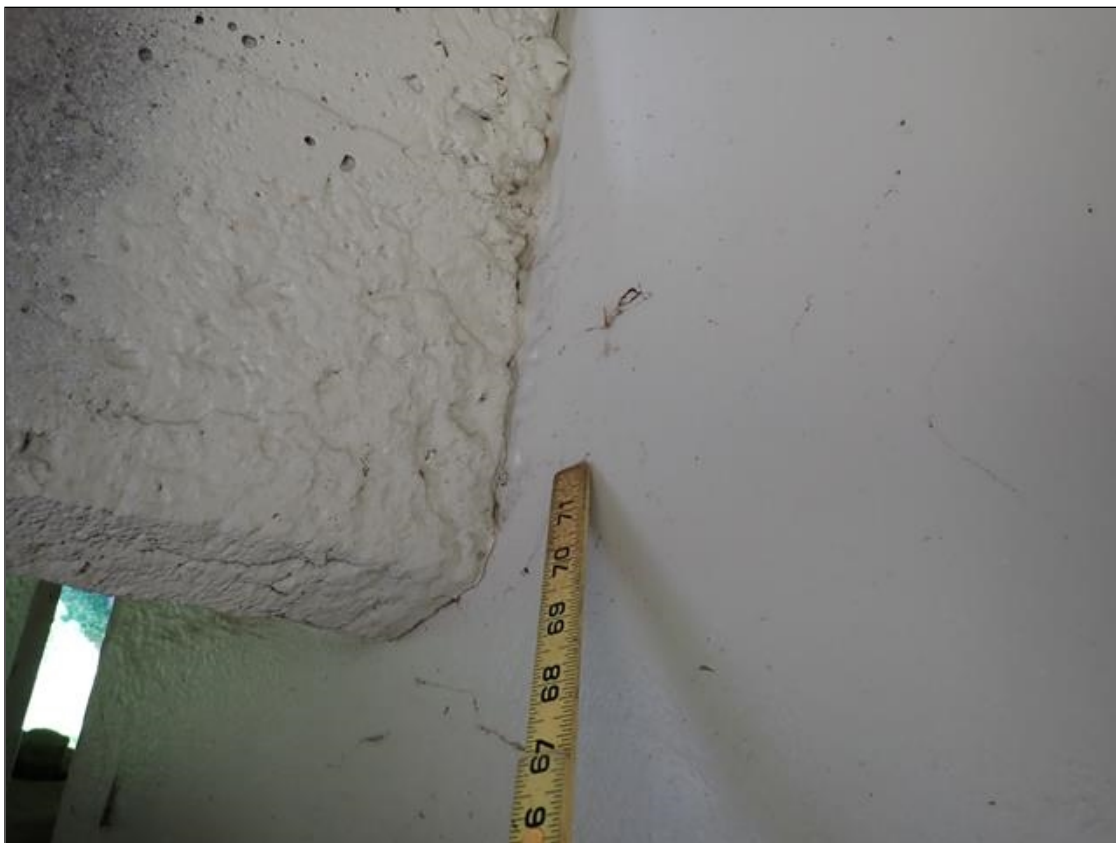
Span 4 Beam 3: at bent 3, web adjacent to end diaphragm, painted over section loss (1/2 inch average remaining x 8 inch x 8 inch)
