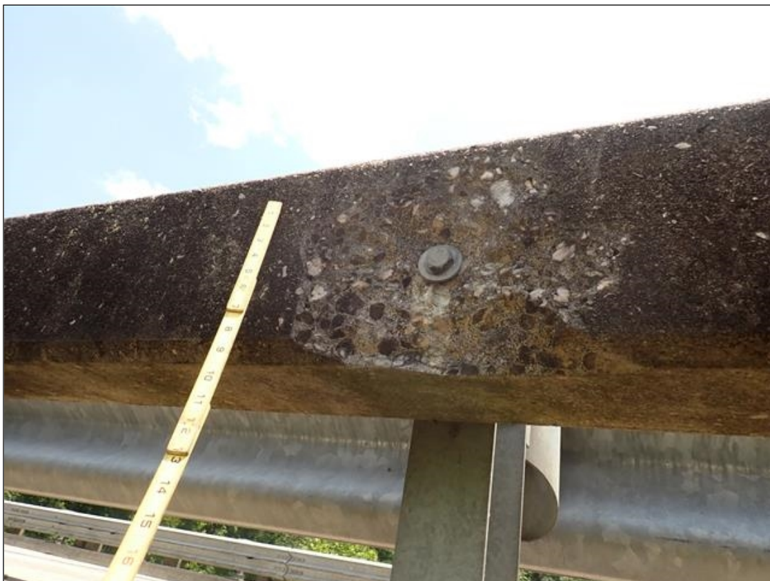
Span 1 Left Bridge Rail: UP TO 8 INCH X 12 INCH X 1.5 INCH DEEP SPALL IN EXTERIOR FACE AT ANCHOR BOLT CONNECTION. TYPICAL AT SEVERAL CONNECTIONS.
