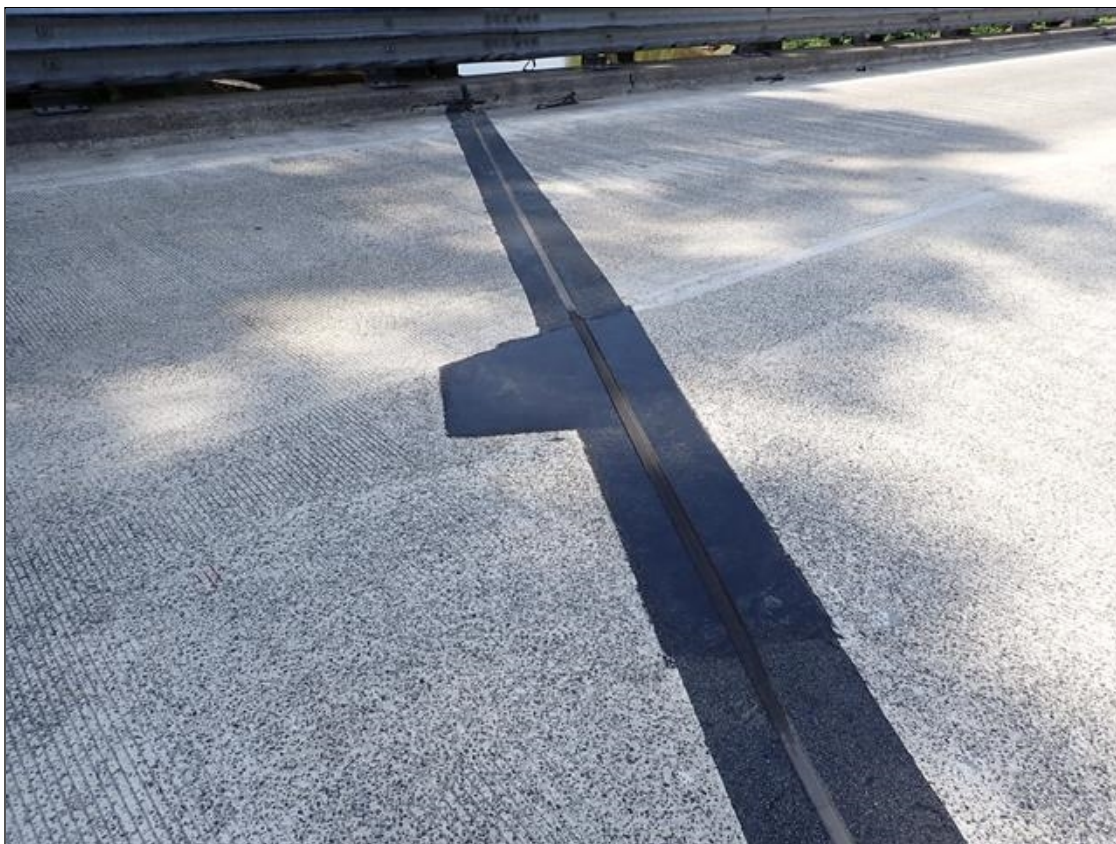
Span 6 Bent 5 Joint: 2025 new repair (29 inch x 21 inch patch), previously noted as: ADJACENT TO DECK SPALL IN SPAN 6, 8 INCHES DIAMETER AREA OF HEADER DEPRESSED BY 1 INCH.
