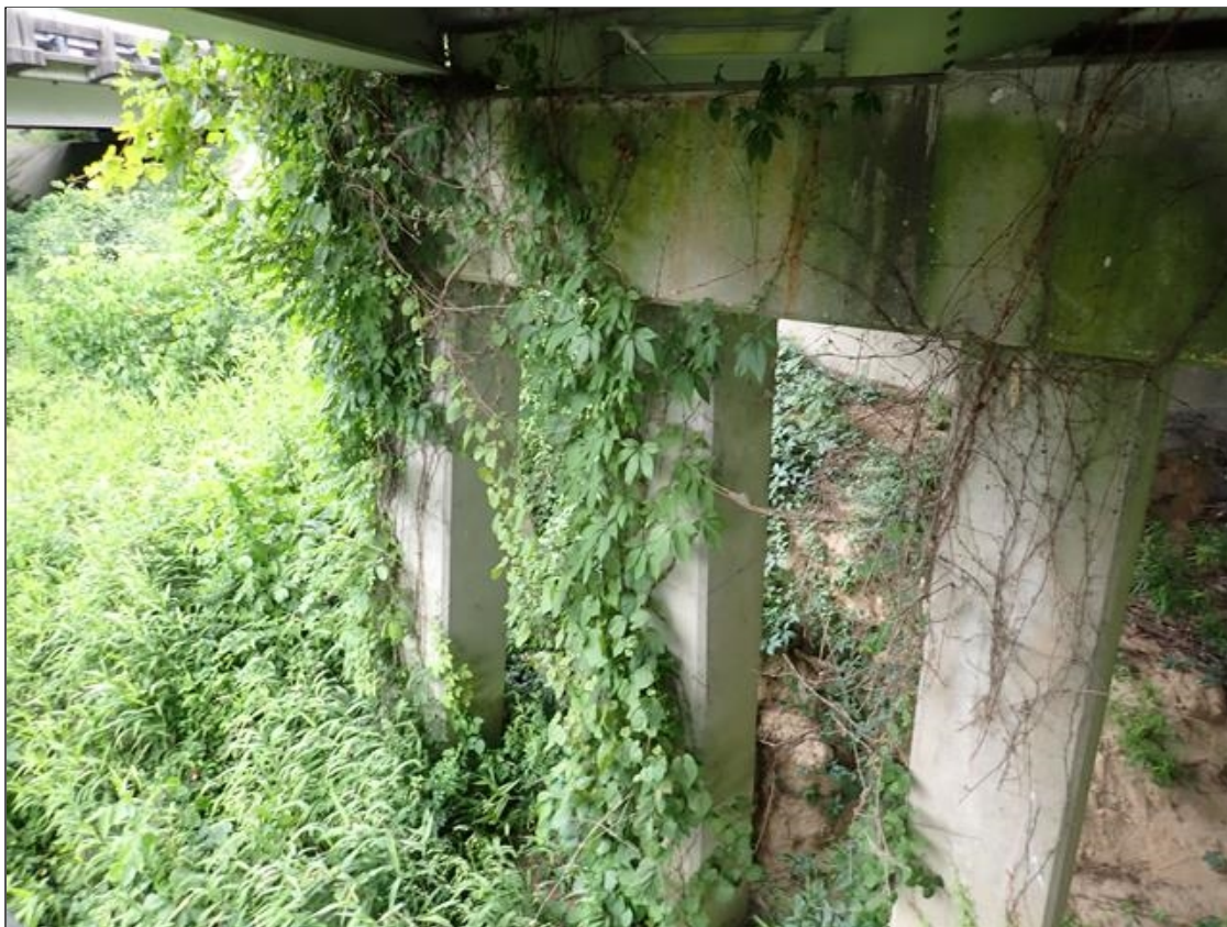
Bent 7 Pile 1: along pile, vegetation growth
