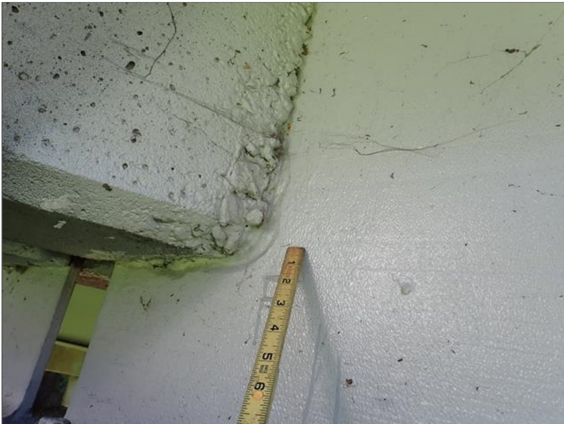
Span 2 Beam 1: at bent 2, web adjacent to end diaphragm, painted over section loss (1/2 inch average remaining x 4 inch x 7 inch)
