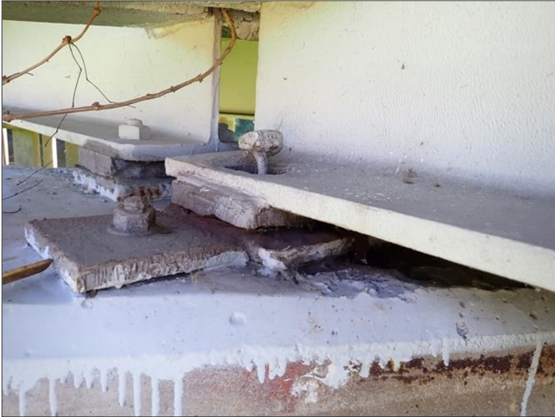
Span 1 Far Bearing 1: LEFT ANCHOR BOLT, PAINTED OVER LOSS (APPROXIMATELY 30 PERCENT REMAINING); WELDED REPAIR, WITH ADDED ANCHOR BOLT.
