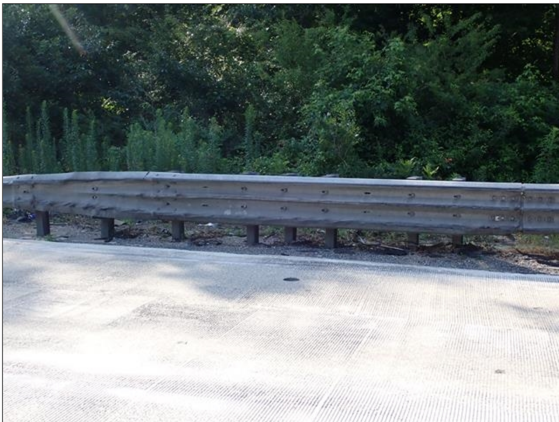
(PAR) northeast guardrail, starting at bridge, impact damage (50 foot)
