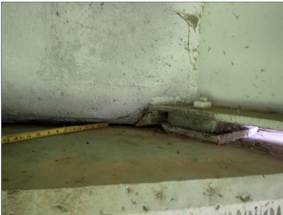
End Bent 1 Abutment: along abutment adjacent to bearings, spalls (up to 12 inch x 6 inch x 2 inch deep)
