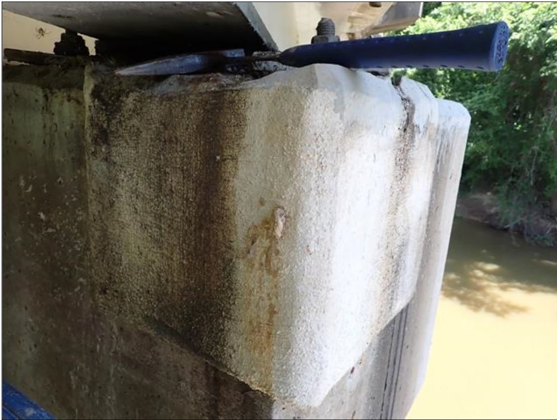
Bent 4 Cap 1: 15 INCHES HIGH X 21 INCHES WIDE SOUND CONCRETE PATCH AREA, TOP SOUTHEAST CORNER OF CAP, BELOW NEW BEARING ASSEMBLY OF BEAM 4.
