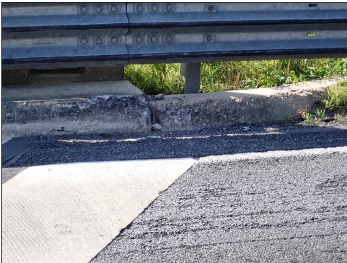
Span 1 Right Bridge Rail: AT END BENT 1, 2 SPALLS IN RAIL AND TOP OF CURB, 1 FOOT LONG X UP TO 4 INCHES X 2 INCHES DEEP
