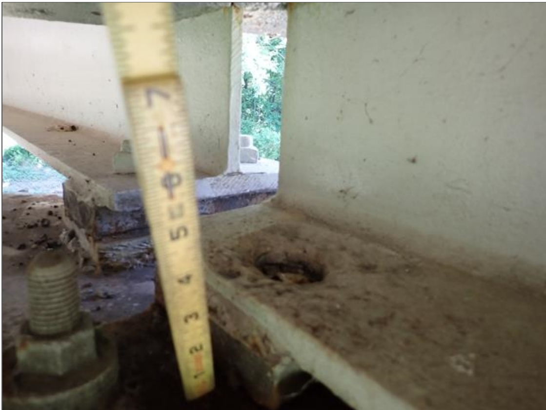
Span 4 Far Bearing 4: BOTH ANCHOR BOLTS ARE MISSING; BEARING ASSEMBLY HAS A WELDED REPAIR WITH NEW ANCHOR BOLTS.
