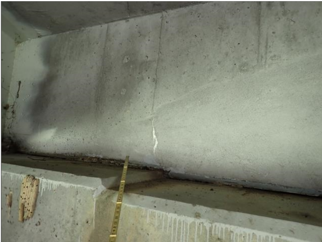
End Bent 1 Abutment: UP TO 3 FEET HIGH X HAIRLINE VERTICAL CRACK WITH EFFLORESCENCE IN BAYS 1 AND 2.
