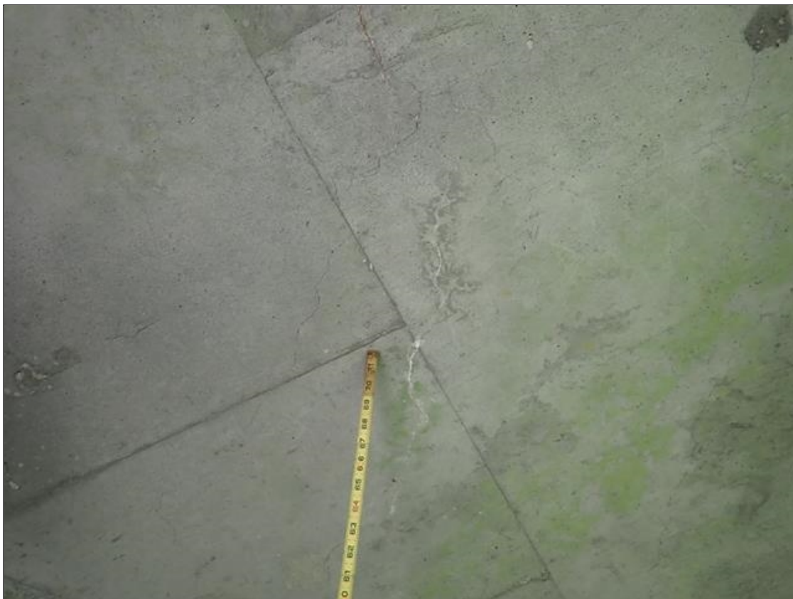
Span 2 Deck: UP TO 0.02 INCH WIDE RANDOM CRACKING SOME WITH EFFLORESCENCE IN DECK UNDERSIDE, SCATTERED THROUGHOUT.
