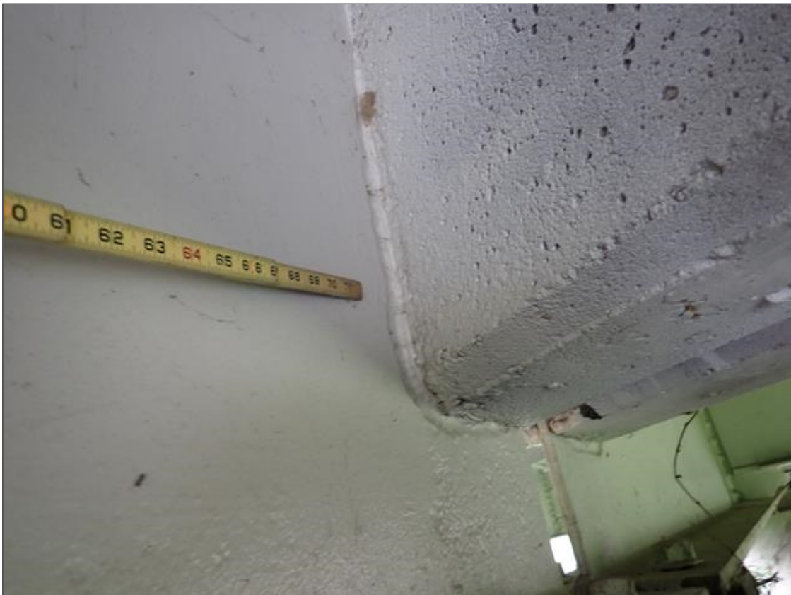
Span 7 Beam 2: (PAR) at bent 7, web adjacent to end diaphragm, painted over section loss (3/8 inch average remaining x 5 inch x 12 inch)
