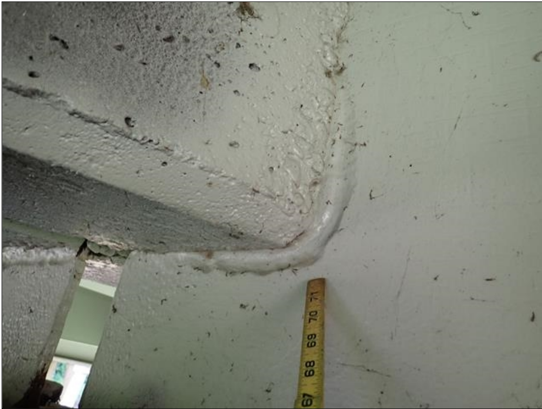
Span 8 Beam 3: (PAR) at bent 7, web adjacent to end diaphragm, painted over section loss (3/8 inch average remaining x 4 inch x 12 inch)
