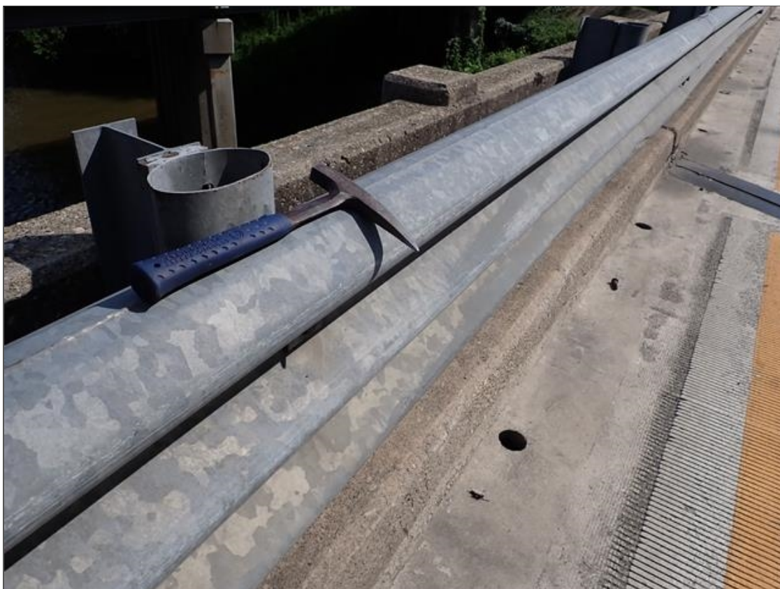
Span 6 Left Retrofit Bridge Rail: near bent 6, impact scrapes (10 foot)
