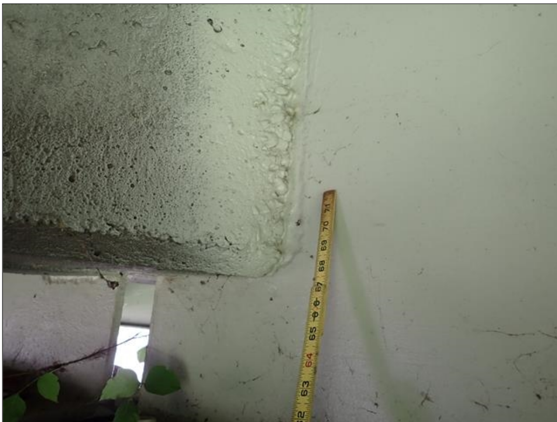
Span 2 Beam 2: (PAR) at bent 1, web adjacent to end diaphragm, painted over section loss (3/8 inch average remaining x 1 inch x 8 inch)
