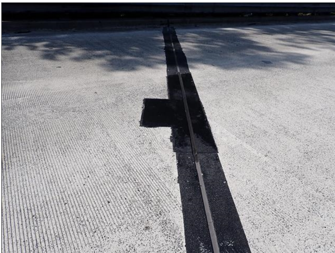
Span 8 Bent 7 Joint: in left travel lane near centerline, patch (28 inch x 18 inch)
