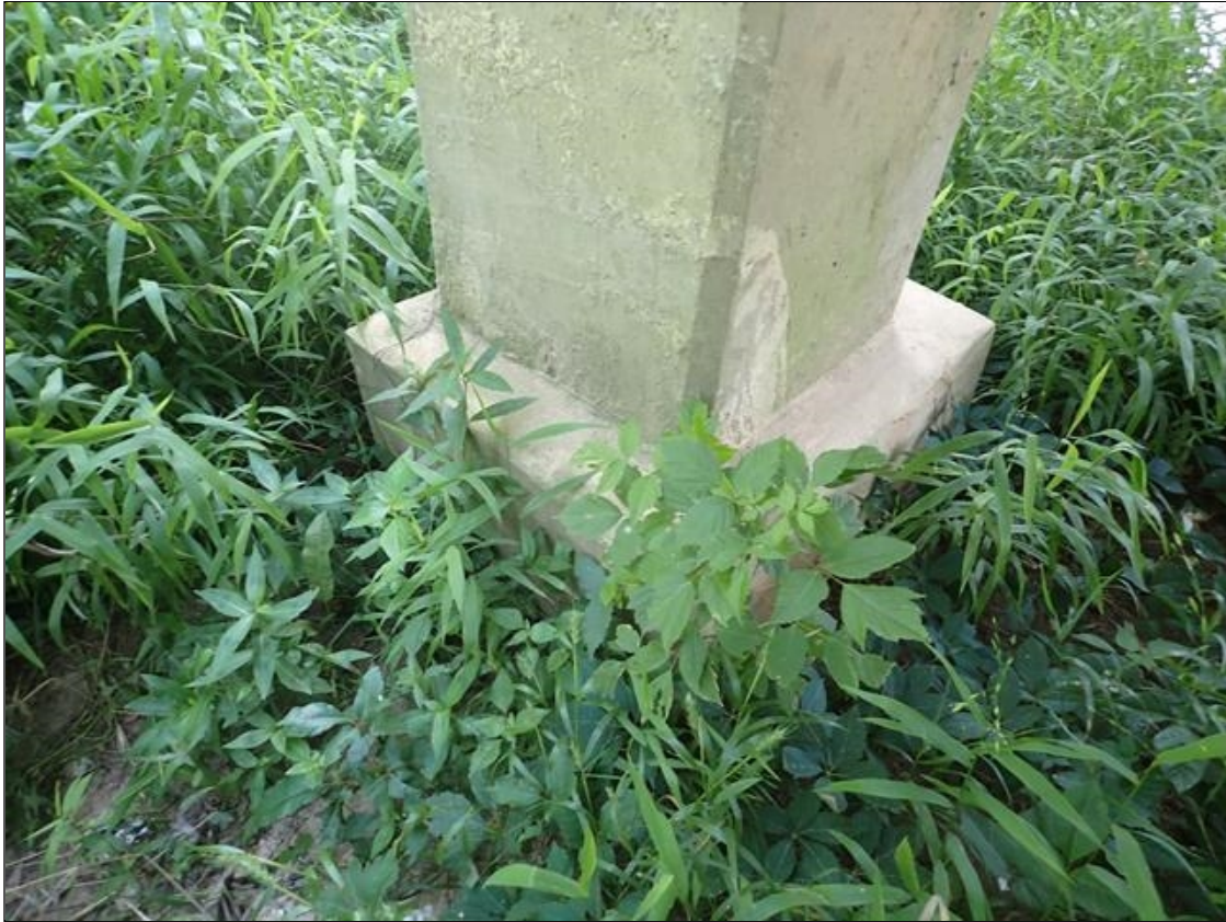
Bent 7 Pile 7: 15 INCHES WIDE X 10 INCHES HIGH AREA OF THE SOUTH FLANGE EXHIBITS SURFACE CORROSION WITH SECTION LOSS ON WEB AND FLANGES OF EXPOSED STEEL PILE AT GROUNDLINE. UP TO 0.50 INCH SECTION REMAINING. NORTH FLANGE AND THE WEB EXHIBIT SURFACE CORROSION WITH NO MEASUREABLE SECTION LOSS. CONCRETE REPAIR AT BASE OF PILE COVERS STEEL PILE.
