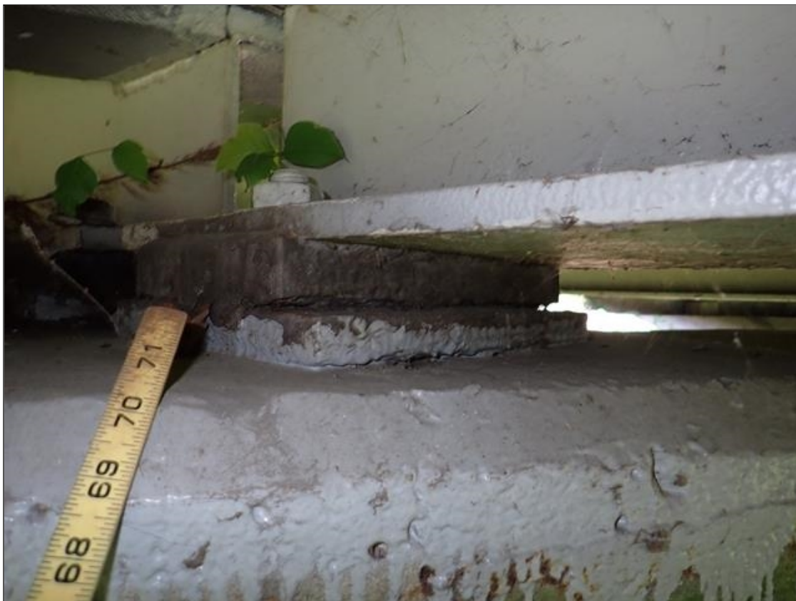
Span 2 Near Bearing 1: painted over section loss (approximately 80 percent remaining)
