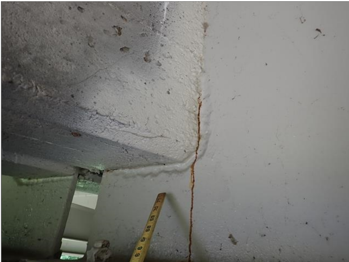
Span 6 Beam 2: (PAR) at bent 6, web adjacent to end diaphragm, painted over section loss (3/8 inch average remaining x 7 inch x 10 inch) with corrosion reactivating
