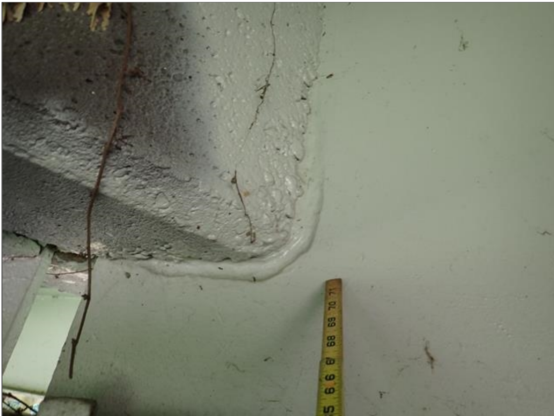
Span 8 Beam 2: (PAR) at bent 7, web adjacent to end diaphragm, painted over section loss (3/8 inch average remaining x 6 inch x 10 inch)
