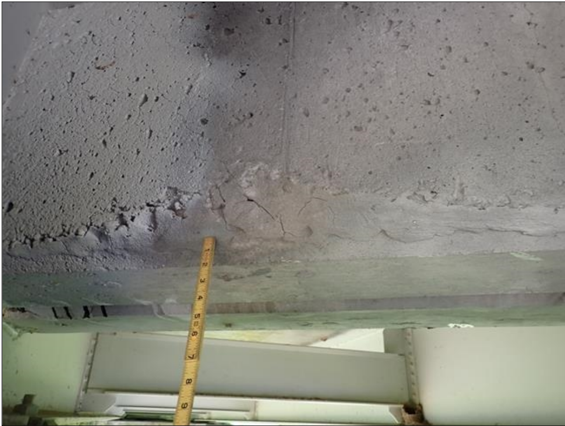
Span 6 Deck: 38 INCHES LONG X 1 FOOT HIGH UNSOUND CONCRETE PATCHED AREA WITH CRACKS (UP TO 1/32 INCH), BOTTOM OF BAY 2 END DIAPHRAGM, AT BENT 6.
