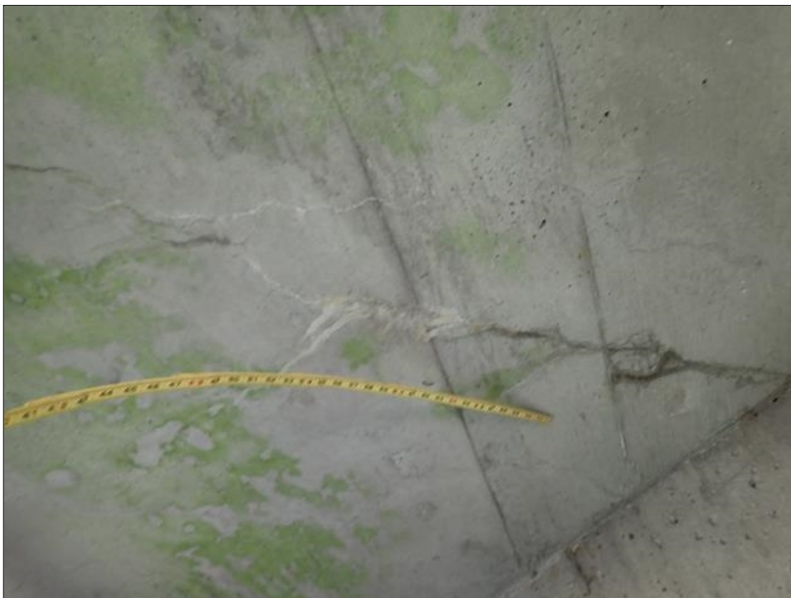
Span 1 Deck: UP TO 0.02 INCH WIDE TRANSVERSE CRACKS SOME WITH EFFLORESCENCE IN DECK UNDERSIDE IN BAY 1 BETWEEN INTERMEDIATE DIAPHRAGMS TYPICAL IN BAYS 2 AND 3.
