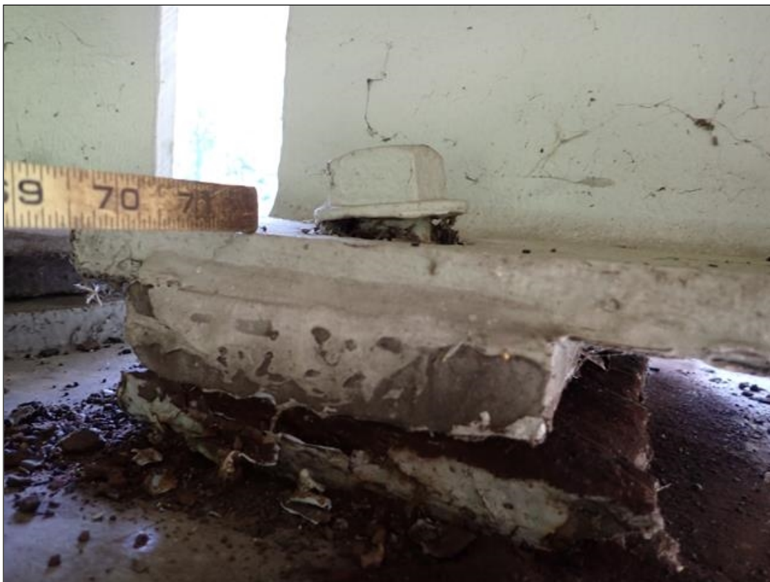
Span 1 Far Bearing 4: left anchor bolt, bent to the north
