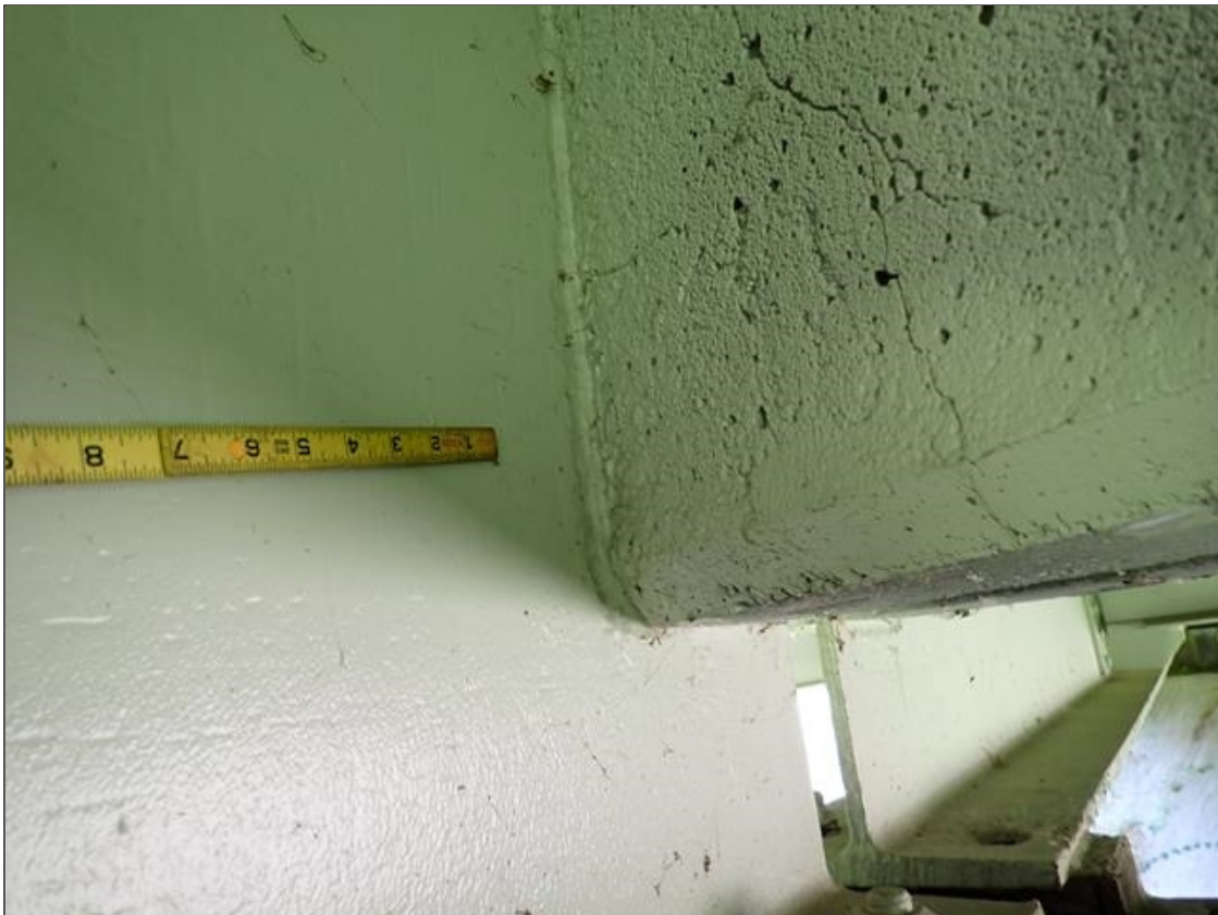
Span 2 Beam 3: at bent 1, web adjacent to end diaphragm, painted over section loss (1/2 inch average remaining x 1 inch x 9 inch)
