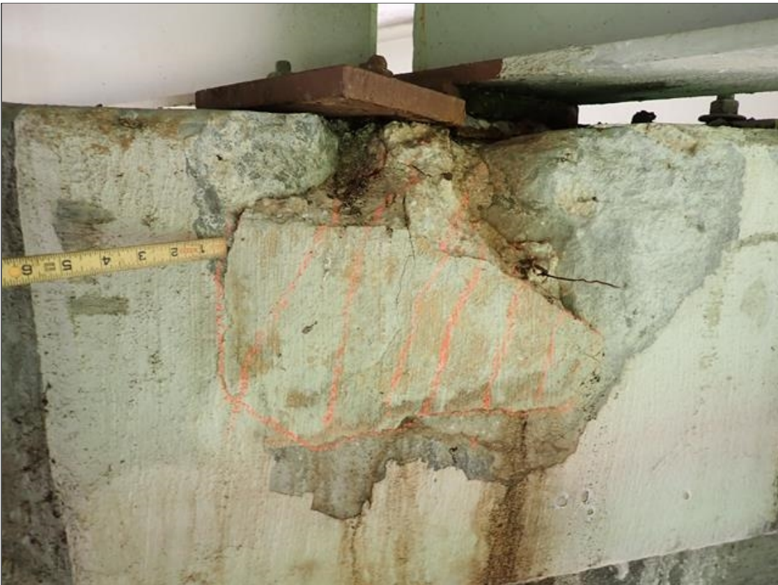
Bent 4 Cap 1: (PAR) SOUTH FACE BELOW BEAM 3 UNSOUND PATCHED AREA WITH SPALLING 4 FEET X 18 INCHES, SPALLS 20 INCHES X 13 INCHES X 6 INCHES DEEP; UNDERMINING BEARING (4 INCH DEEP)
