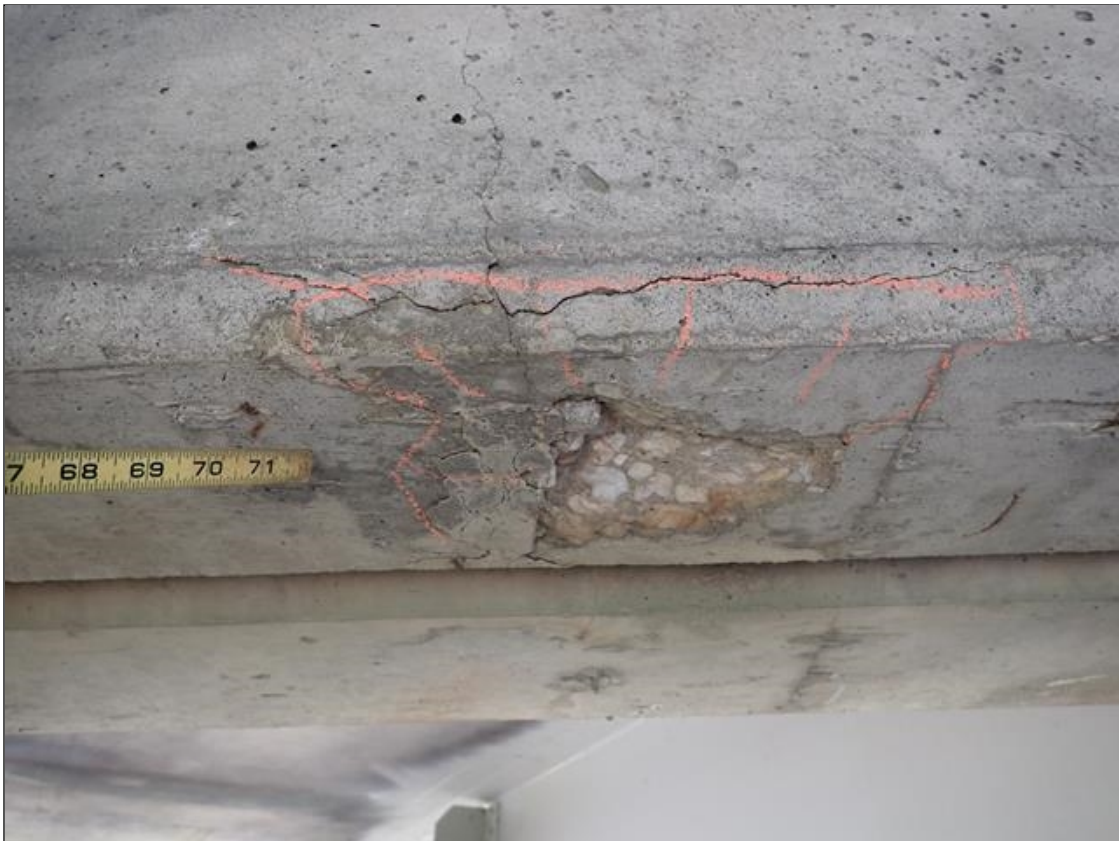
Span 5 Deck: 12 INCHES X 8 INCH X 3/4 INCH DEEP SPALL/DELMINATION IN INTERMEDIATE DIAPHRAGM IN BAY 2 ABOVE BENT 5.
