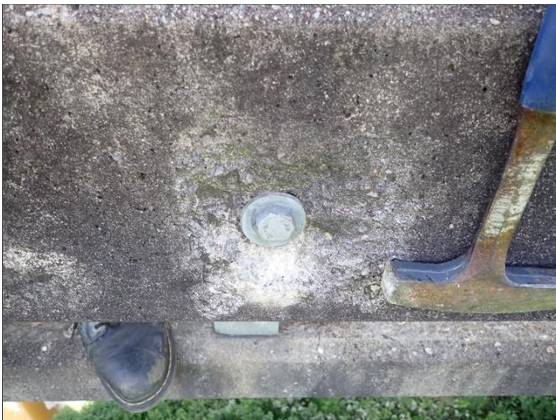
Span 3 Left Bridge Rail: UP TO 6 INCH DIAMETER X 1.5 INCH DEEP SPALL IN EXTERIOR FACE AT ANCHOR BOLT CONNECTION. TYPICAL AT SEVERAL CONNECTIONS.
