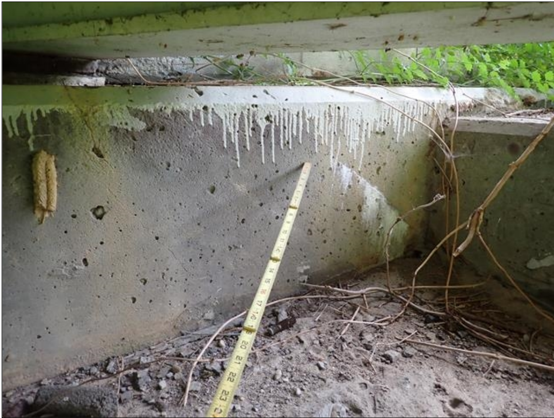
End Bent 1 Cap 1: FOUR (4) DIAGONAL X FULL HEIGHT HAIRLINE CRACKS SOME WITH EFFLORESCENCE IN FACE OF CAP BELOW BAY 1.
