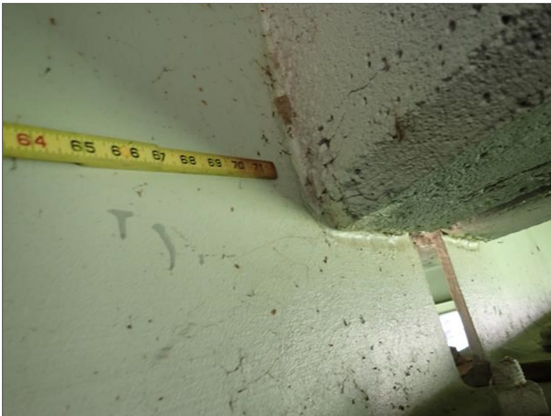
Span 3 Beam 2: at bent 2, web adjacent to end diaphragm, painted over section loss (9/16 inch average remaining x 7 inch x 2 inch)
