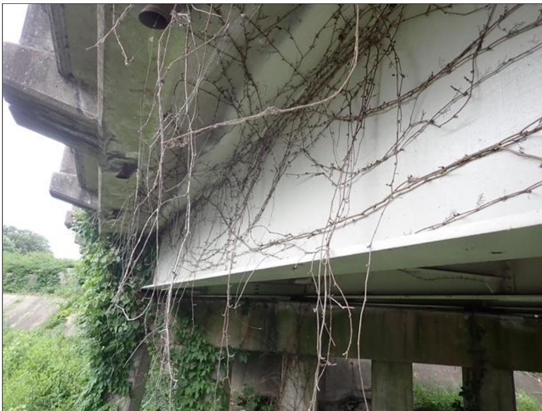
Span 7 Beam 1: along beam, vegetation growth
