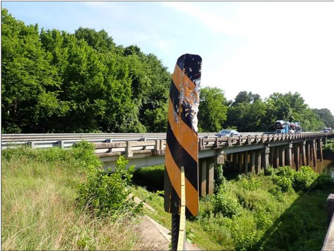
Span 1 Southwest Delineator: (PAR) IMPACT DAMAGE TO SIGN WITH SCRAPING AND DISTORTIONS.
