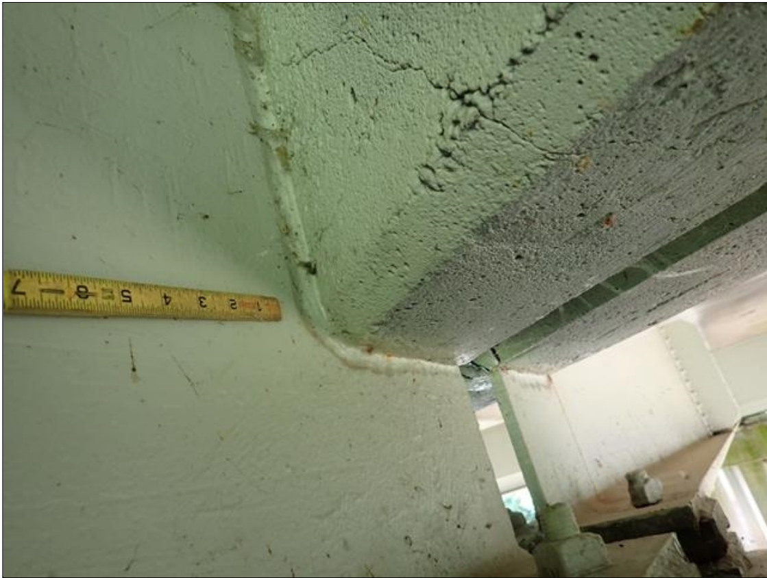
Span 7 Beam 2: (PAR) at bent 6, web adjacent to end diaphragm, painted over section loss (3/8 inch average remaining x 7 inch x 14 inch) with corrosion reactivating
