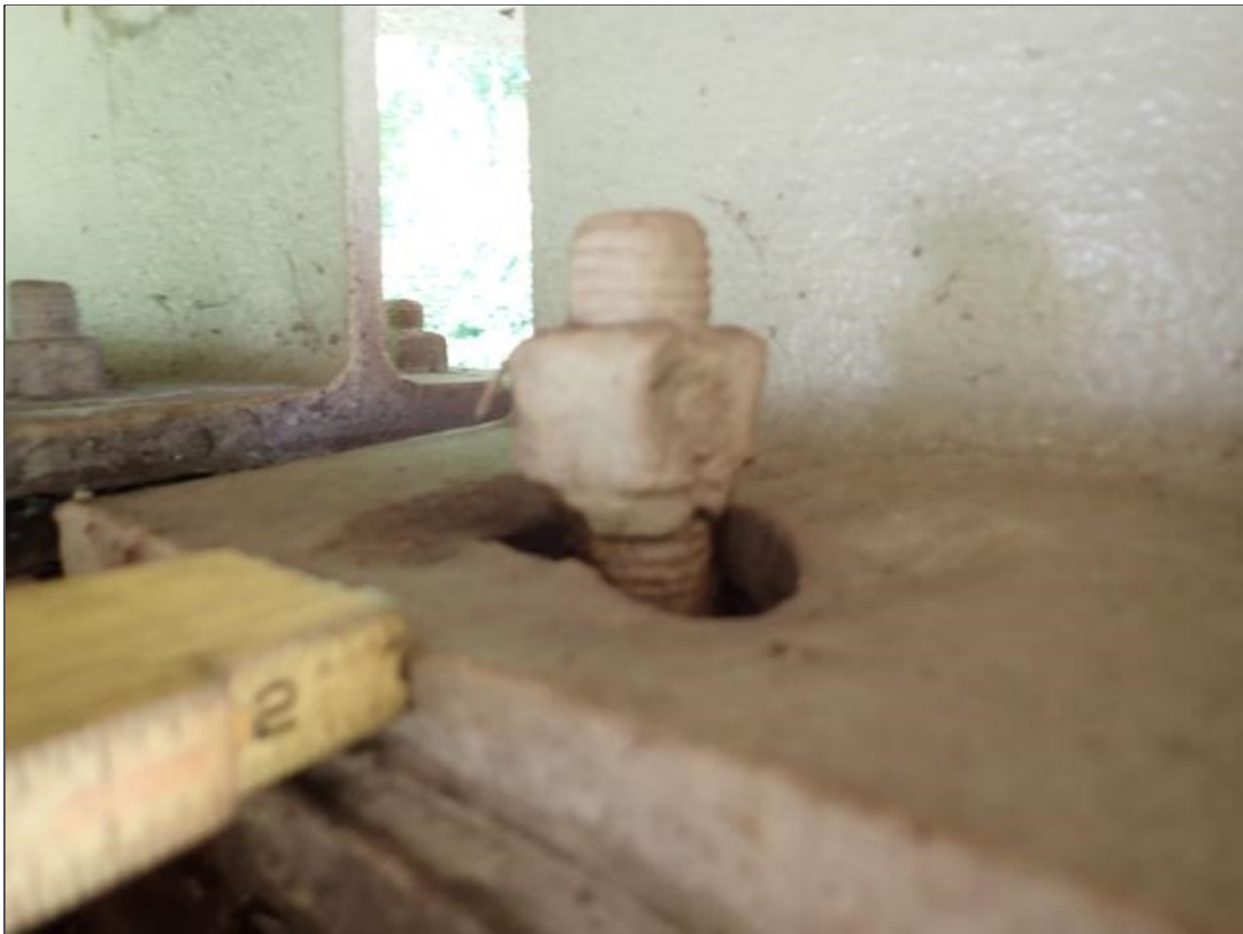
Span 6 Far Bearing 4: corrosion with section loss (approximately 80 percent remaining); left anchor bolt nut, painted over loss (approximately 80 percent remaining)
