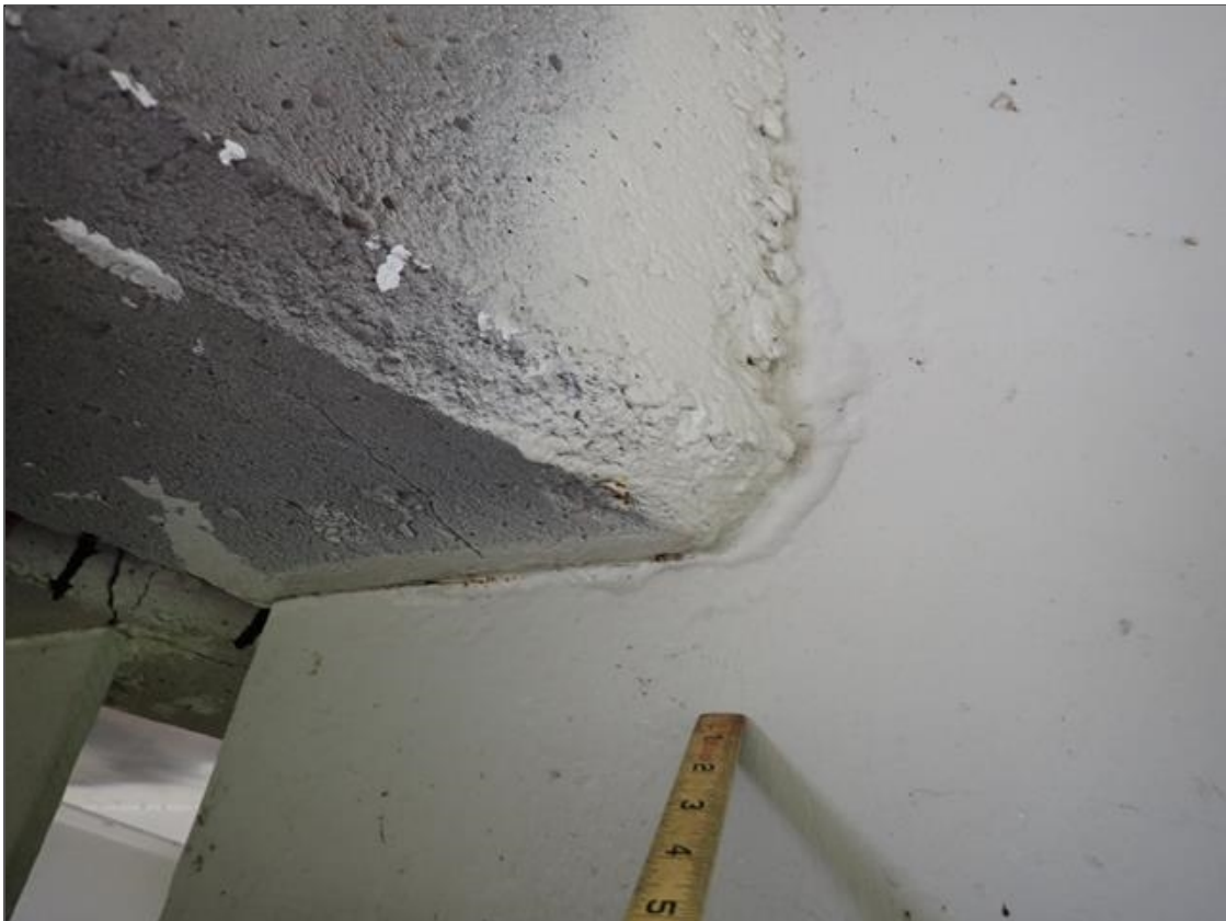
Span 5 Beam 2: (PAR) at bent 5, web adjacent to end diaphragm, painted over section loss (3/8 inch average remaining x 10 inch x 1 inch) with corrosion reactivating
