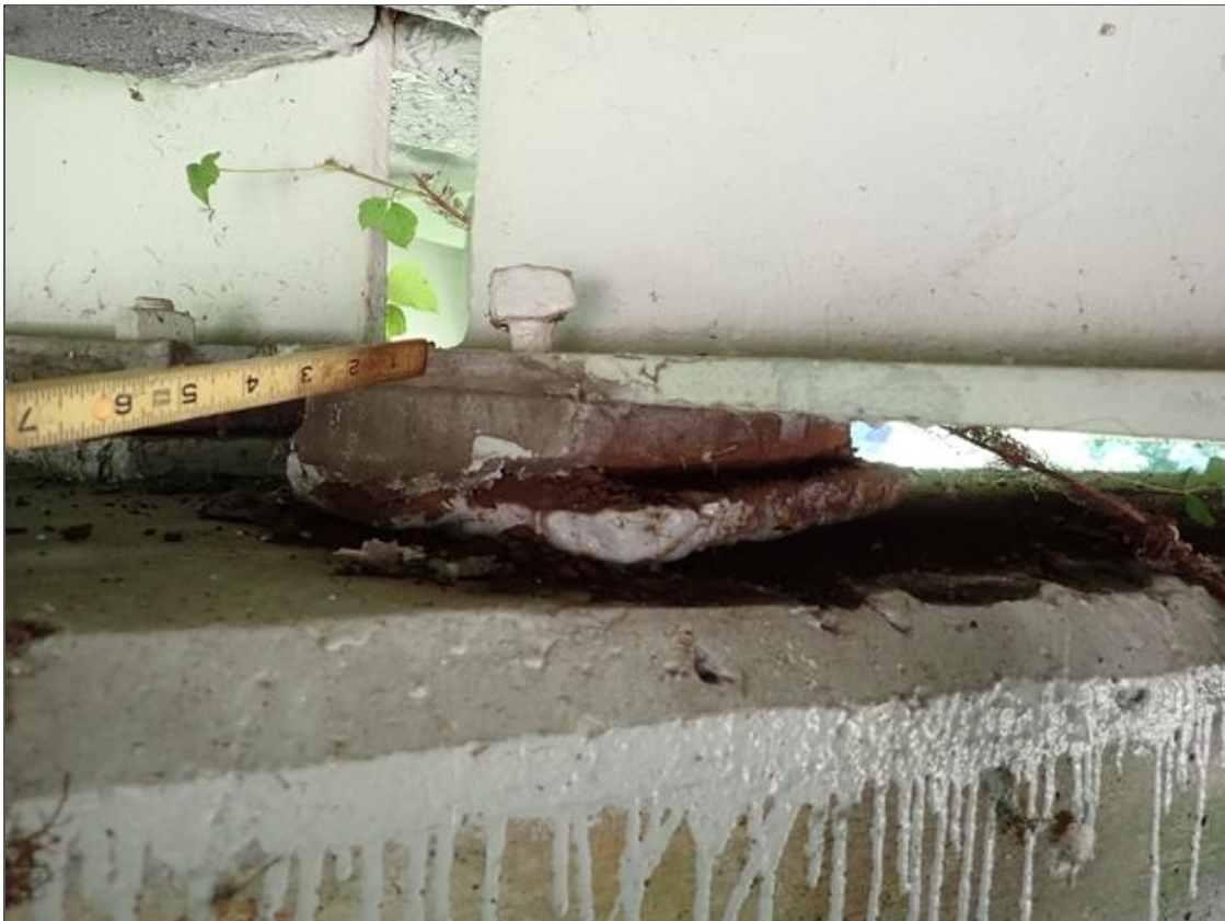
Span 1 Far Bearing 2: (PAR) painted over section loss (approximately 80 percent remaining); left anchor bolt, painted over section loss (approximately 50 percent remaining)
