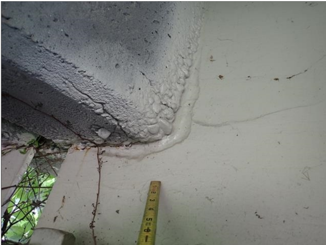
Span 8 Beam 1: (PAR) at bent 7, web adjacent to end diaphragm, painted over section loss (3/8 inch average remaining x 4 inch x 10 inch) with corrosion reactivating
