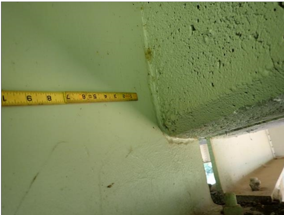
Span 7 Beam 3: (PAR) at bent 6, web adjacent to end diaphragm, painted over section loss (3/8 inch average remaining x 7 inch x 12 inch) with corrosion reactivating
