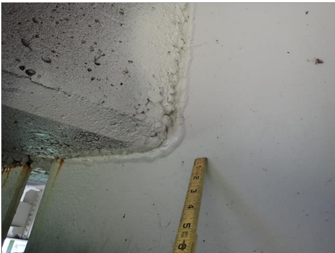
Span 5 Beam 2: (PAR) at bent 4, web adjacent to end diaphragm, painted over section loss (3/8 inch average remaining x 8 inch x 18 inch) with corrosion reactivating
