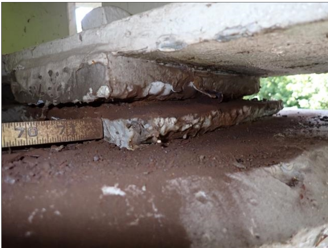
Span 1 Far Bearing 4: painted over section loss (approximately 80 percent remaining)
