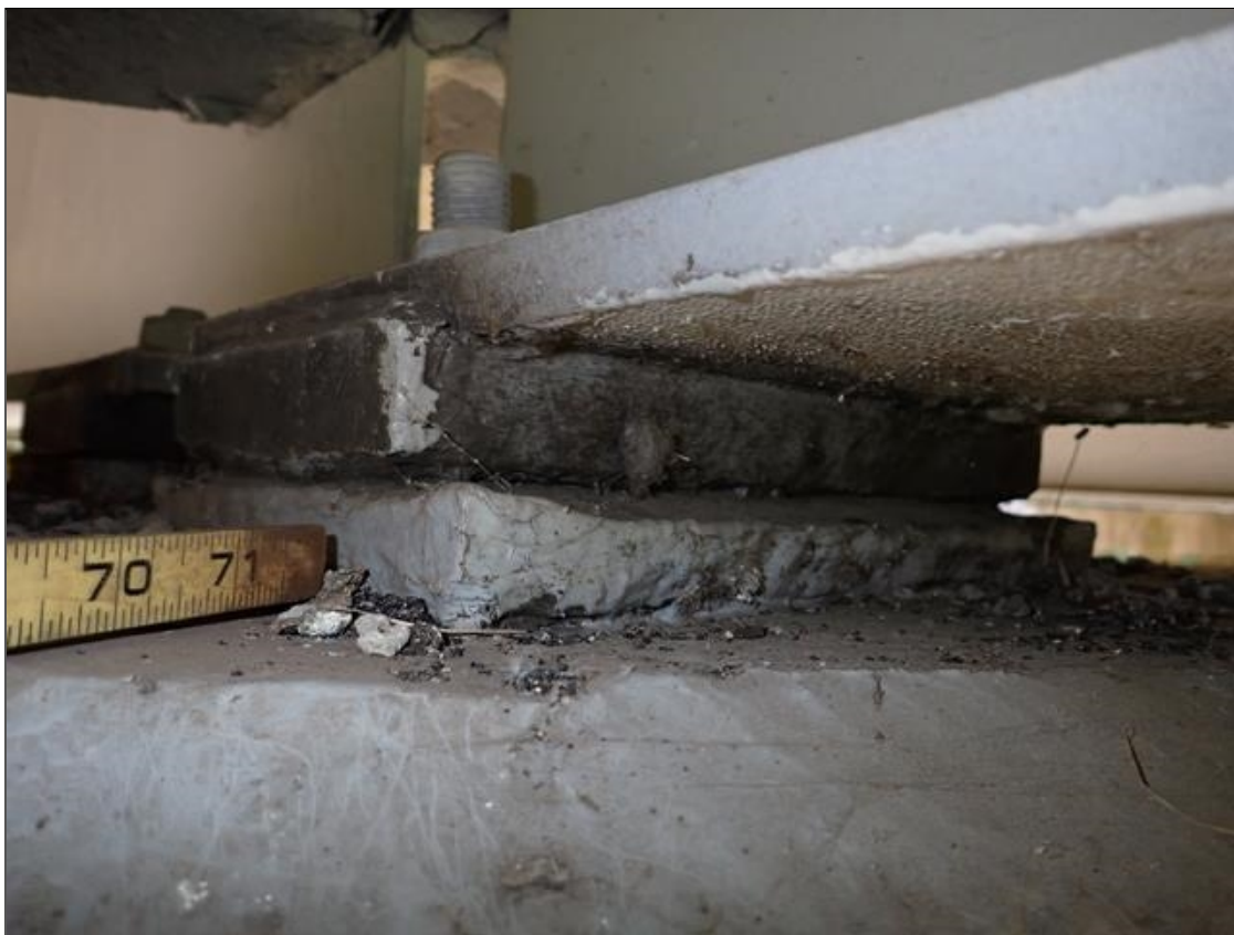
Span 6 Near Bearing 2 : painted over section loss (approximately 80 percent remaining)
