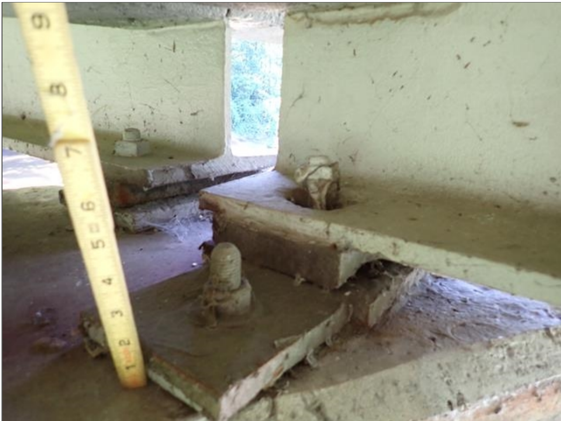
Span 2 Far Bearing 1: WELDED REPAIR WITH NEW ANCHOR BOLT. UP TO 50 PERCENT SECTION LOSS IN OLD ANCHOR BOLT. PAR NOT ISSUED DUE TO NEW ANCHOR BOLT REPAIR.
