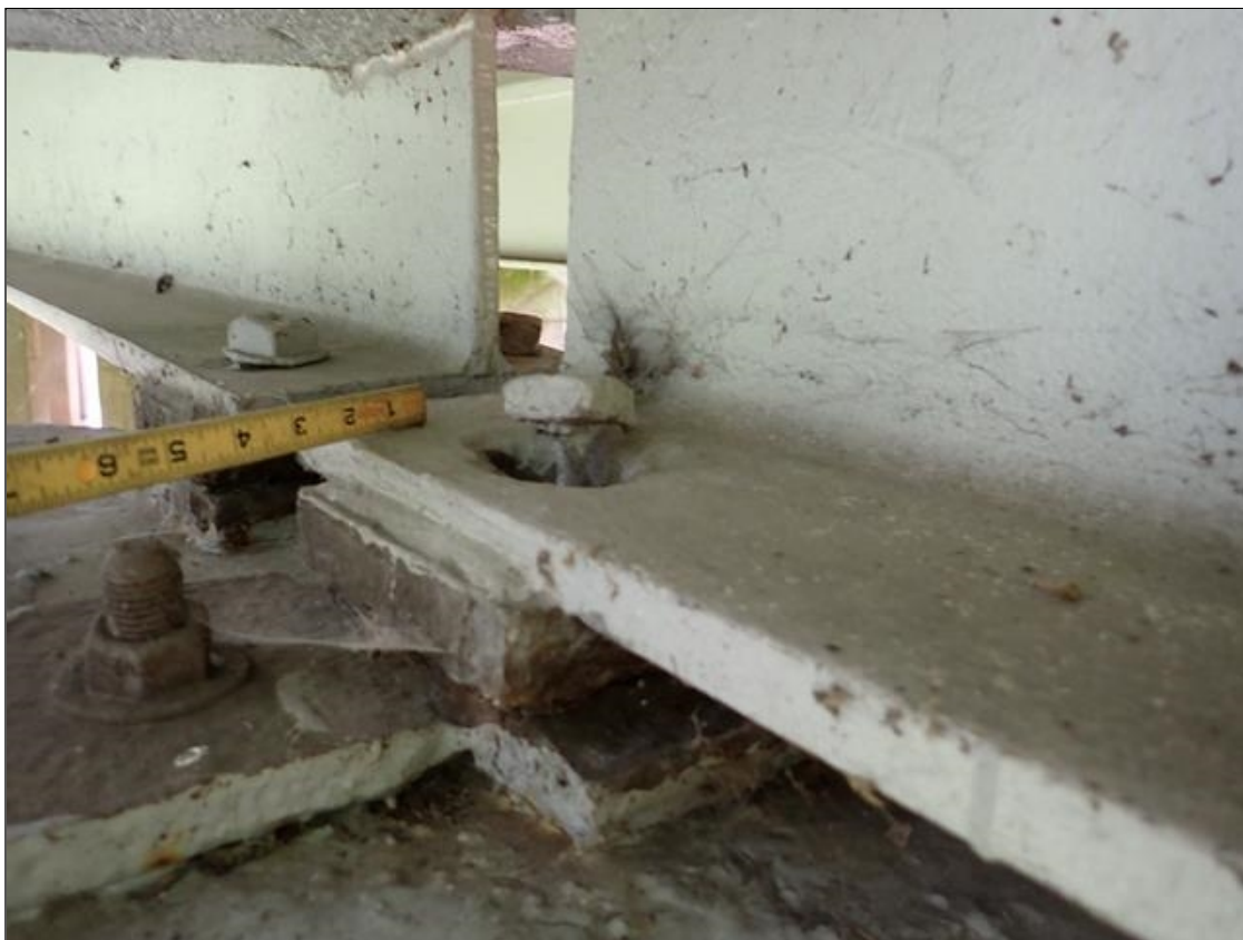
Span 8 Near Bearing 4: (PAR) right anchor bolt, painted over section loss (approximately 25 percent remaining); previous repair in place
