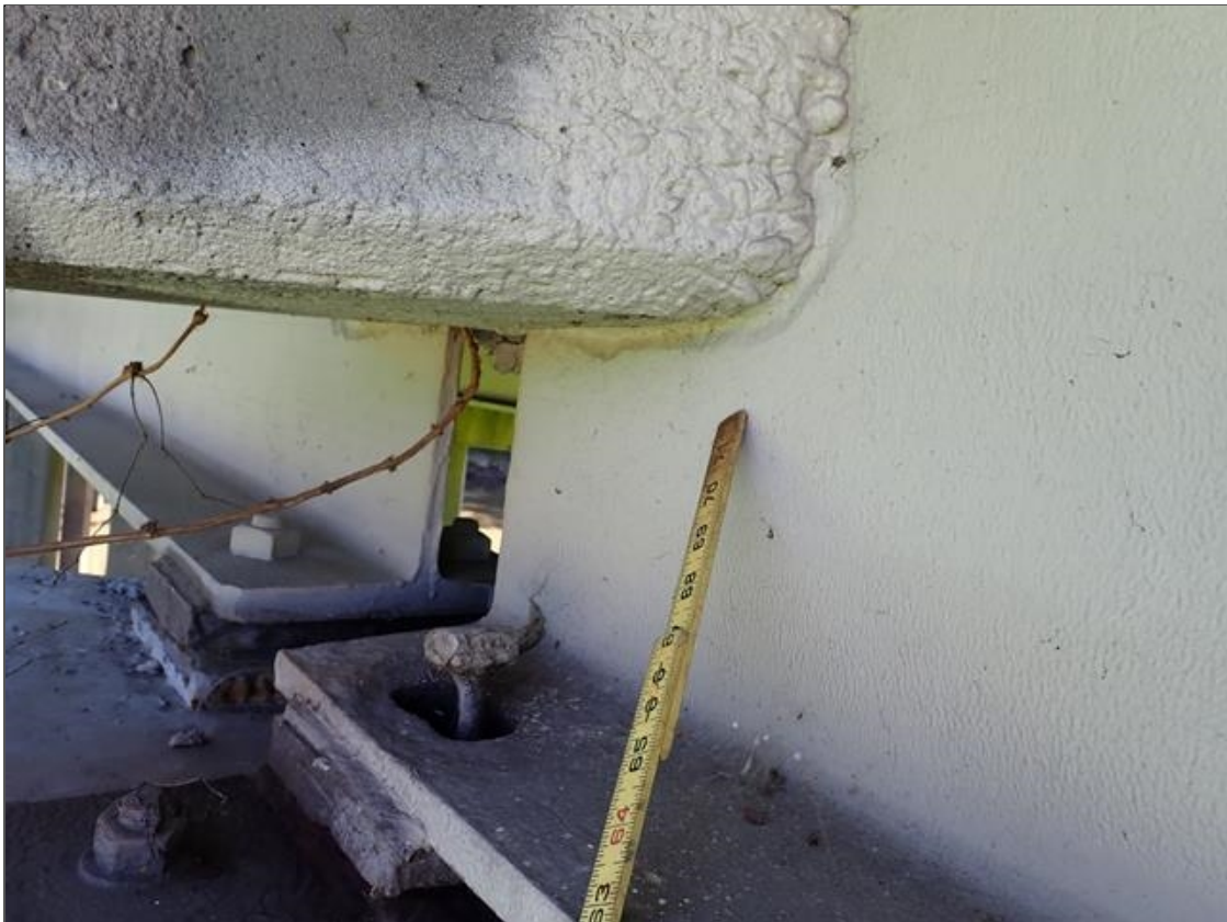
Span 1 Beam 1: (PAR) at bent 1, painted over section loss: web adjacent to end diaphragm (3/8 inch average remaining x 3 inch x 18 inch); bottom flange (less than 1/16 inch loss x 4 diameter)
