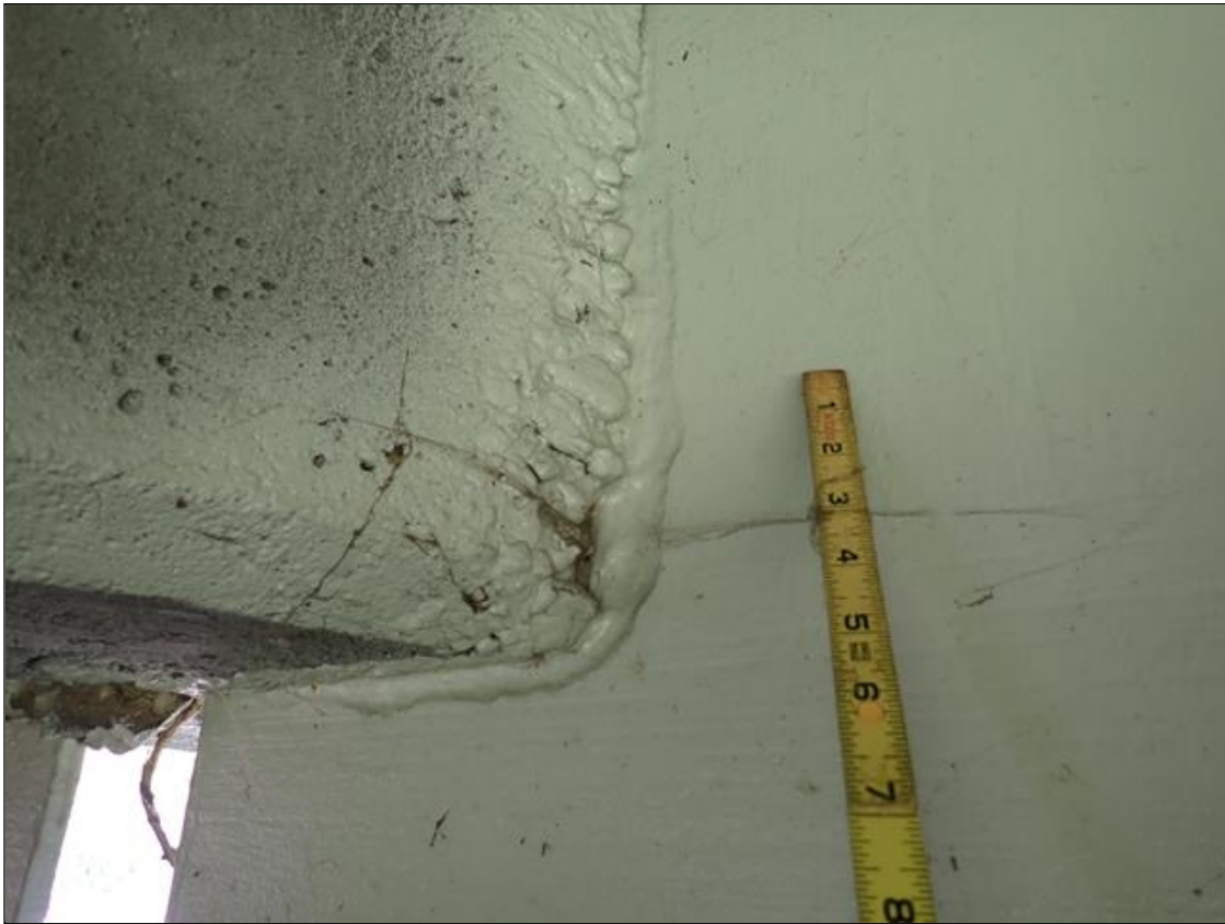
Span 2 Beam 1: (PAR) at bent 1, web adjacent to end diaphragm, painted over section loss (3/8 inch average remaining x 7 inch x 9 inch)
