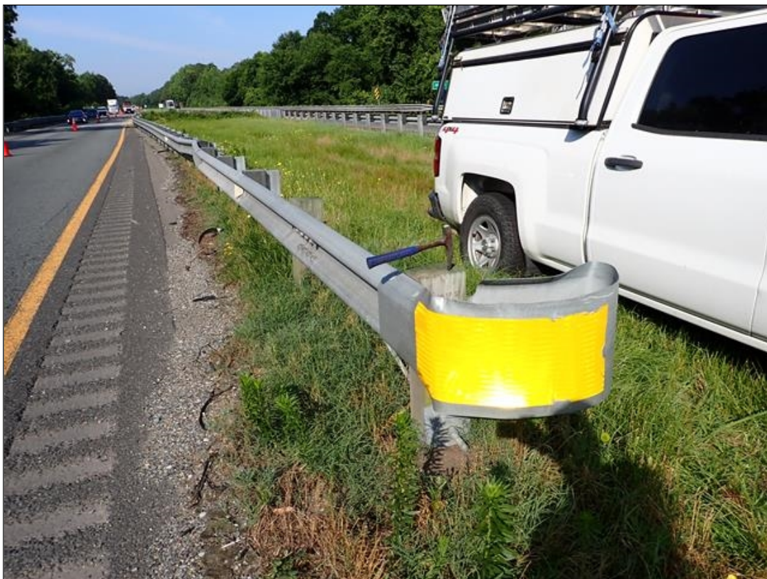
northwest guardrail termination
