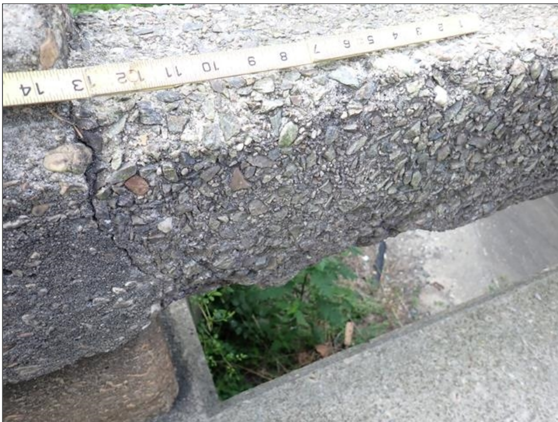
Span 8 Right Bridge Rail: AT END BENT 2, BOTTOM FACE, 1 FOOT LONG X 4 INCHES WIDE X 1 INCH DEEP SPALL
