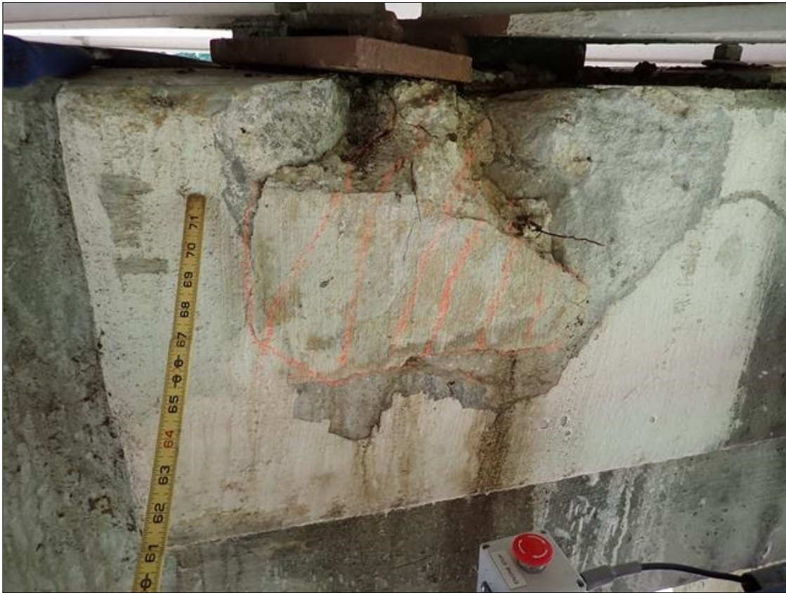
Span 4 Far Bearing 3: (PAR) ADDED BEARING HAS A LOSS OF BEARING AREA DUE TO SPALL ON CAP. AREA REPAIRED IS UNSOUND AND HAS 13 INCHES HIGH X 20 INCHES WIDE X 6 INCHES DEEP SPALL/ DELAMINATION.
