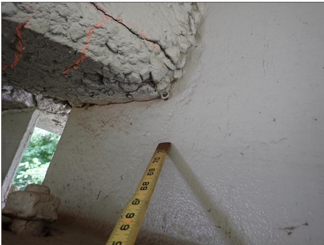
Span 5 Beam 4: at bent 5, painted over pitting (up to 1/16 inch deep x 8 inch x 10 inch)
