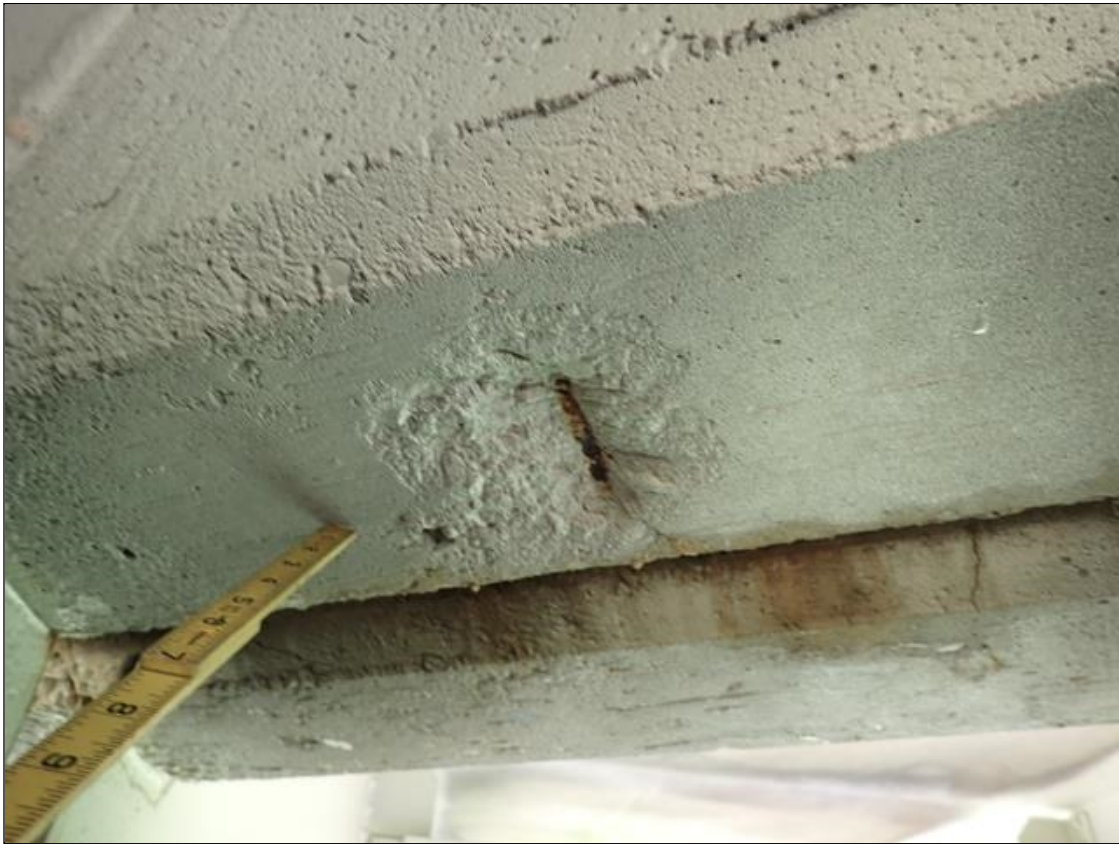
Span 5 Deck: span 5, bay 2 end diaphragm over bent 4, underside, spall (6 inch x 6 inch x 3/4 inch deep) with exposed rusted rebar
