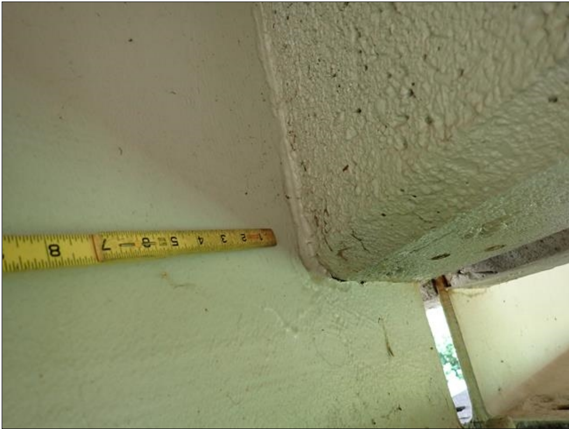
Span 5 Beam 4: (PAR) at bent 4, web adjacent to end diaphragm, painted over section loss (3/8 inch average remaining x 8 inch x 1 inch)
