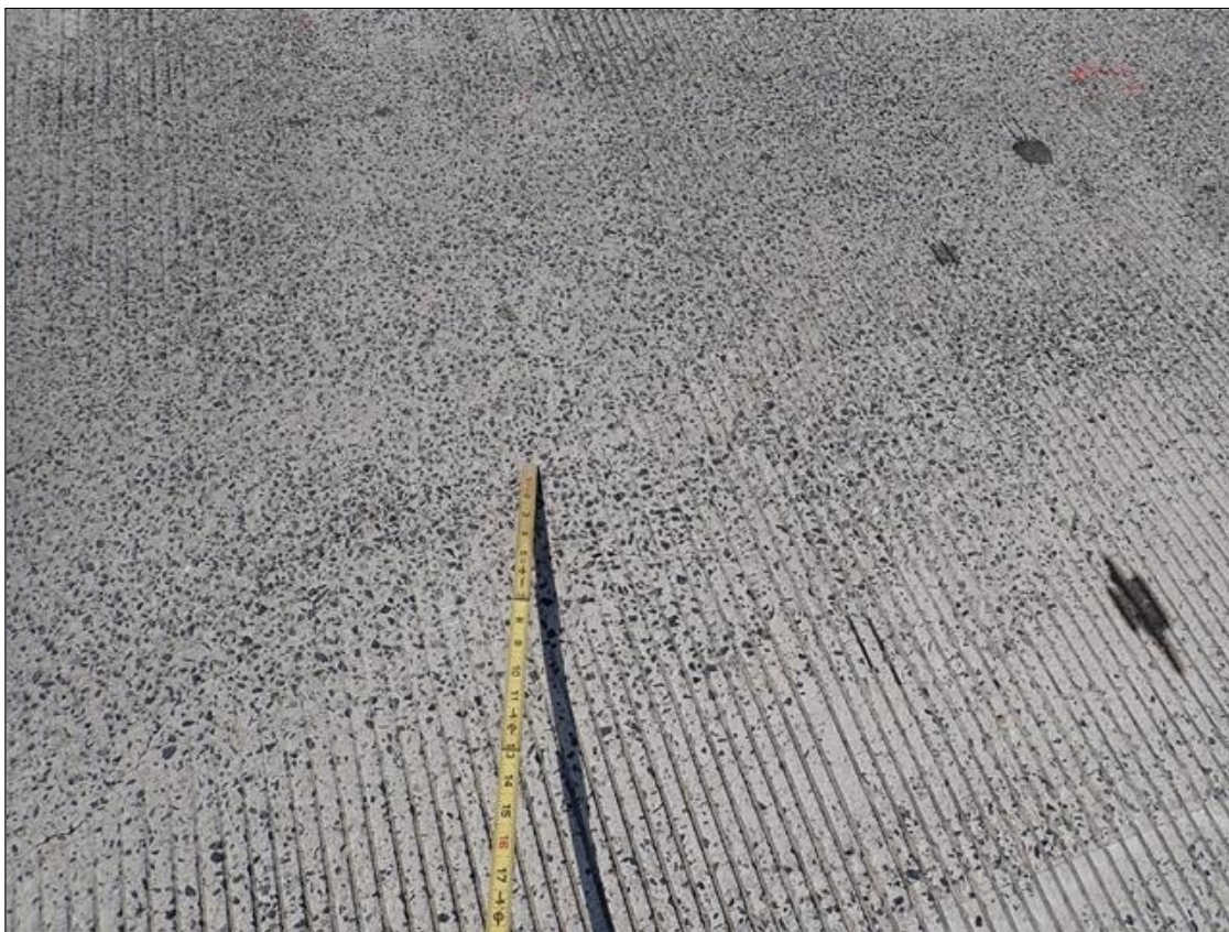
Approach 2: throughout slab, map cracks (hairline) at random
