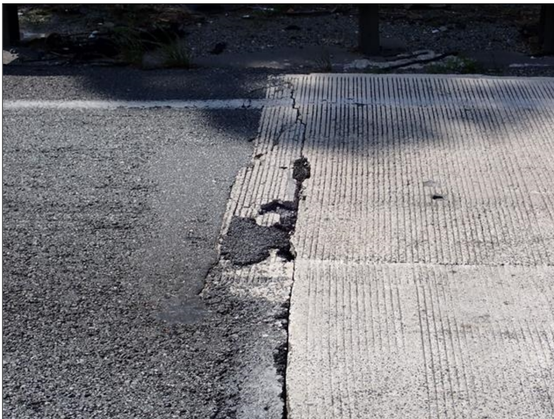
Approach 2: northeast corner, area of broken/cracked concrete (5 foot x 1 foot x 2 inch deep) with settlement (2 inch deep)
