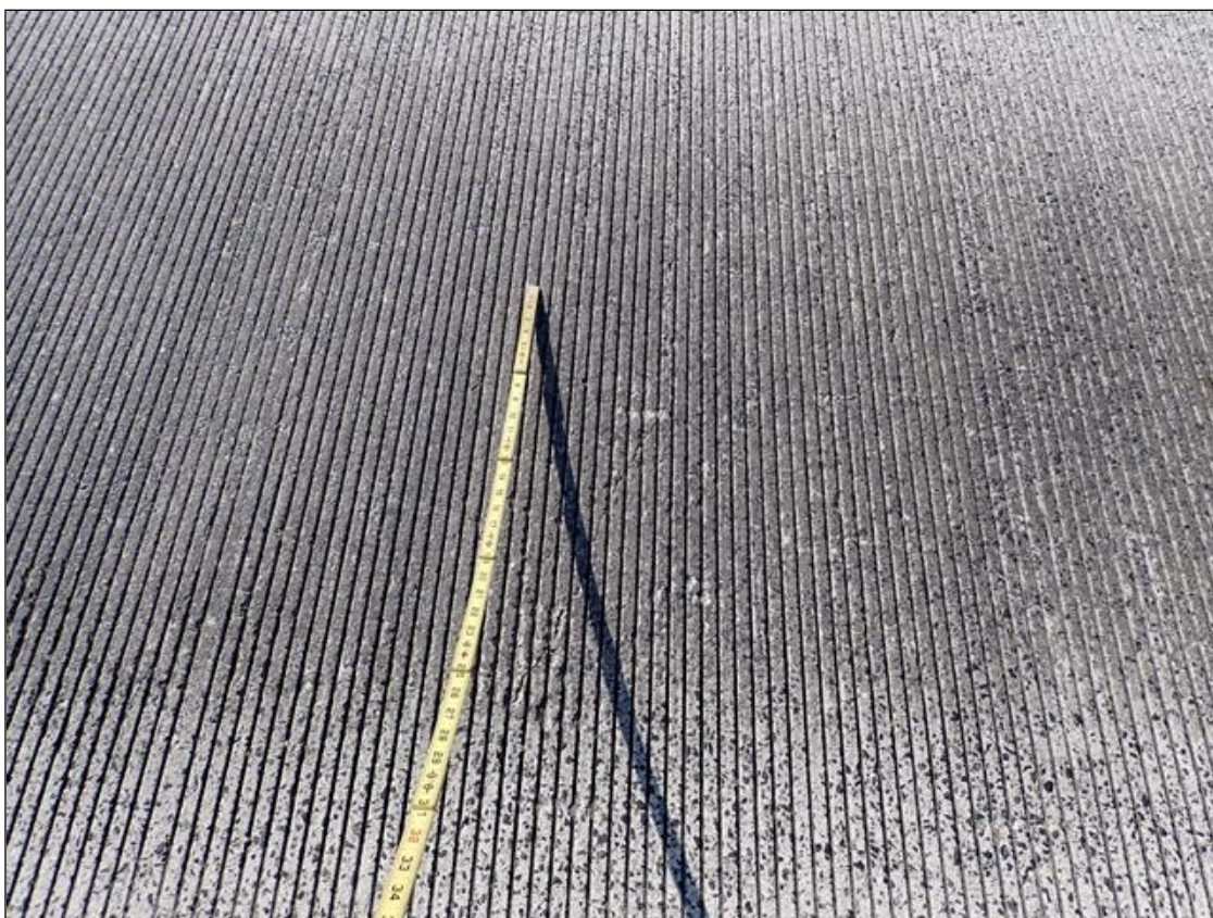
Span 1 Deck: throughout top of deck, areas of map cracks (up to 1/32 inch) at random
