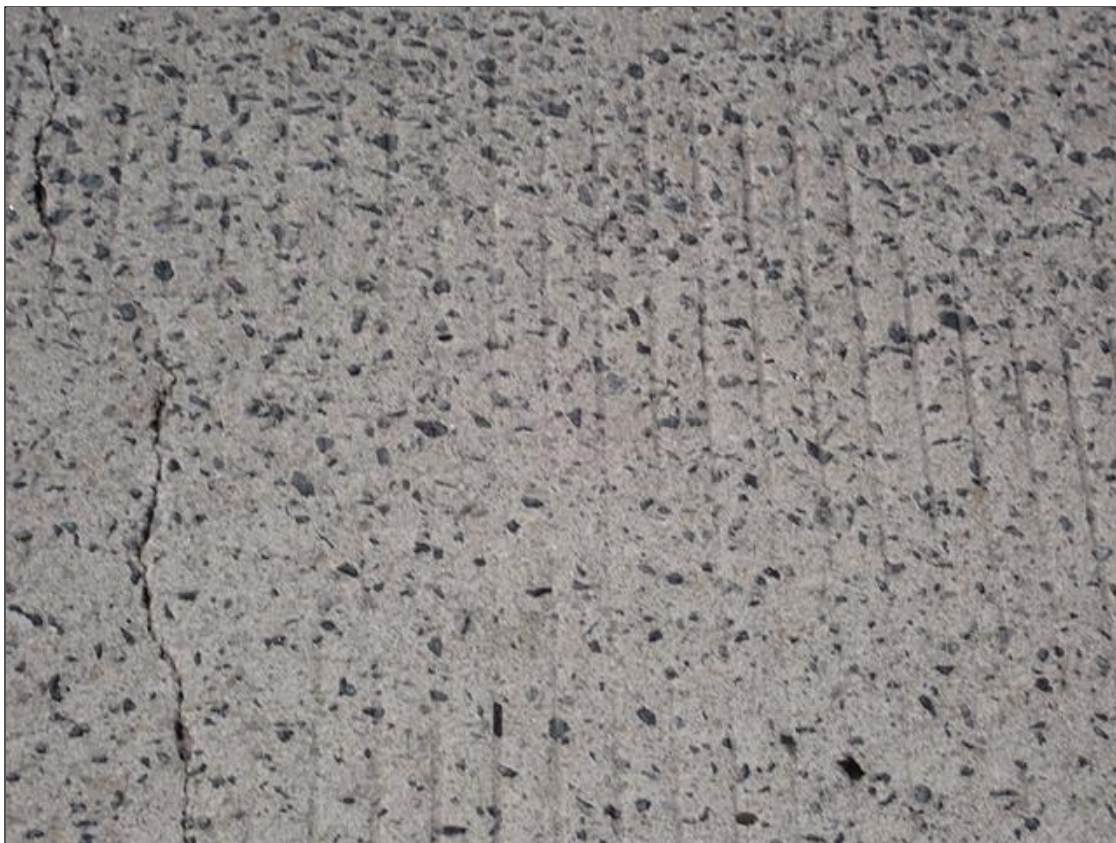
Span 8 Deck: throughout top of deck, areas of map cracks (hairline) and transverse cracks (up to 1/32 inch x 12 foot) at random
