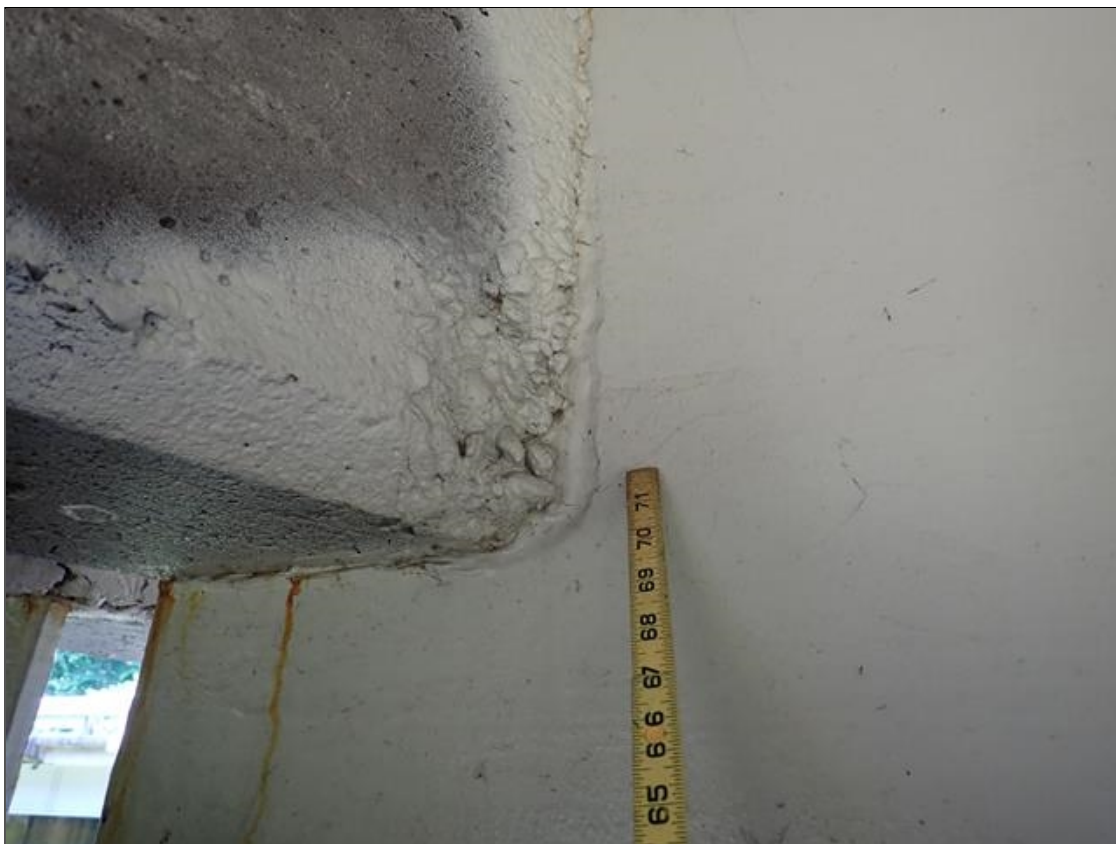
Span 5 Beam 1: (PAR) at bent 4, web adjacent to end diaphragm, painted over section loss (3/8 inch average remaining x 8 inch x 1 inch) with corrosion reactivating
