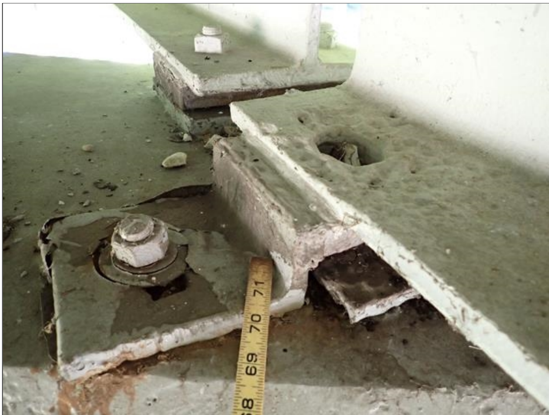
Span 1 Far Bearing 3: LEFT ANCHOR BOLT MISSING; WELDED REPAIR WITH ADDED ANCHOR BOLT.
