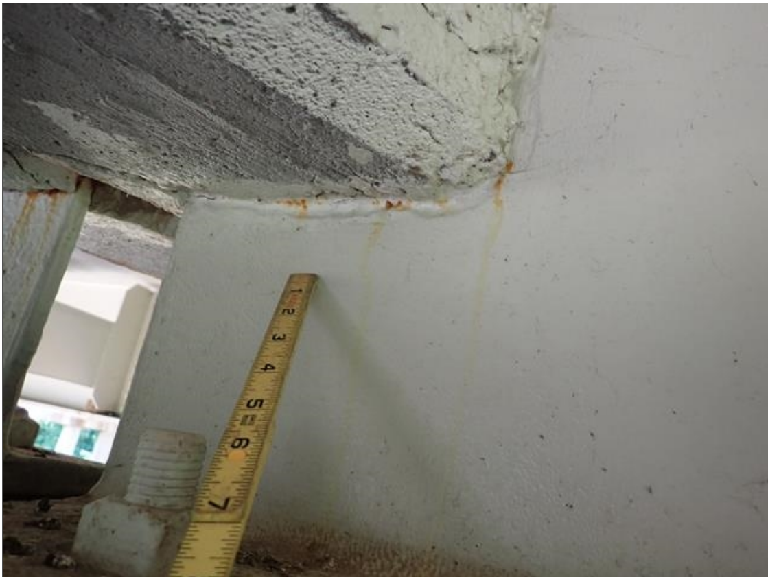
Span 6 Beam 3: at bent 5, web adjacent to end diaphragm, painted over section loss (9/16 inch average remaining x 8 inch x 8 inch) with corrosion reactivating
