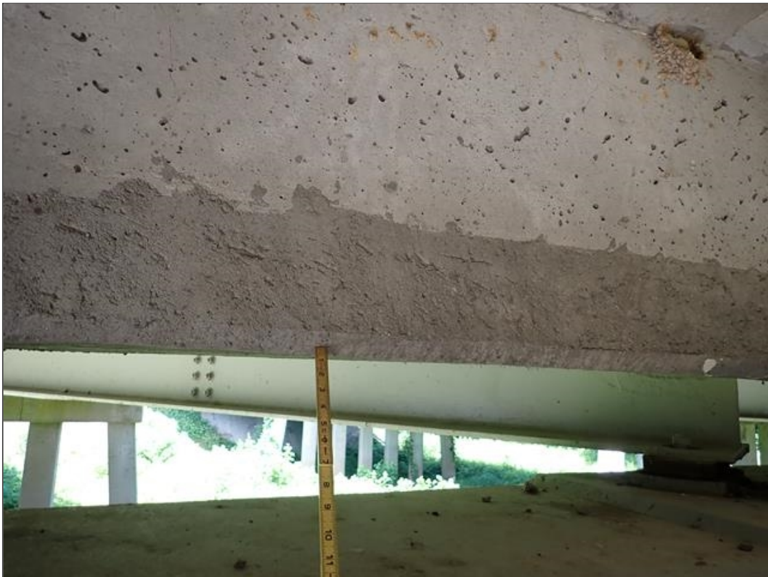
Span 4 Deck: 4 FEET LONG X 1 FOOT HIGH AREA OF UNSOUND CONCRETE PATCH WITH UP TO 1/64 INCH VERTICAL CRACKS IN BAY 3 BENT DIAPHRAGM AT BENT 3.
