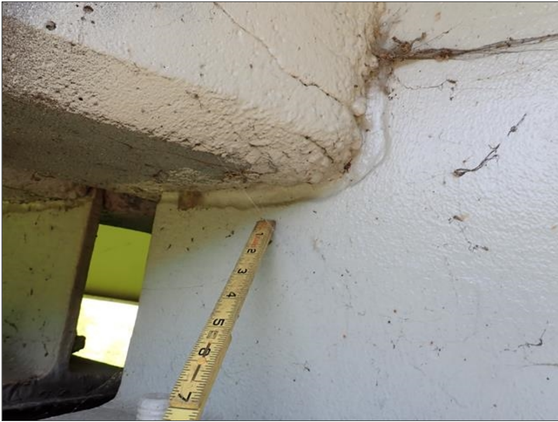
Span 3 Beam 4: at bent 2, web adjacent to end diaphragm, painted over section loss (1/2 inch average remaining x 10 inch x 1 inch)
