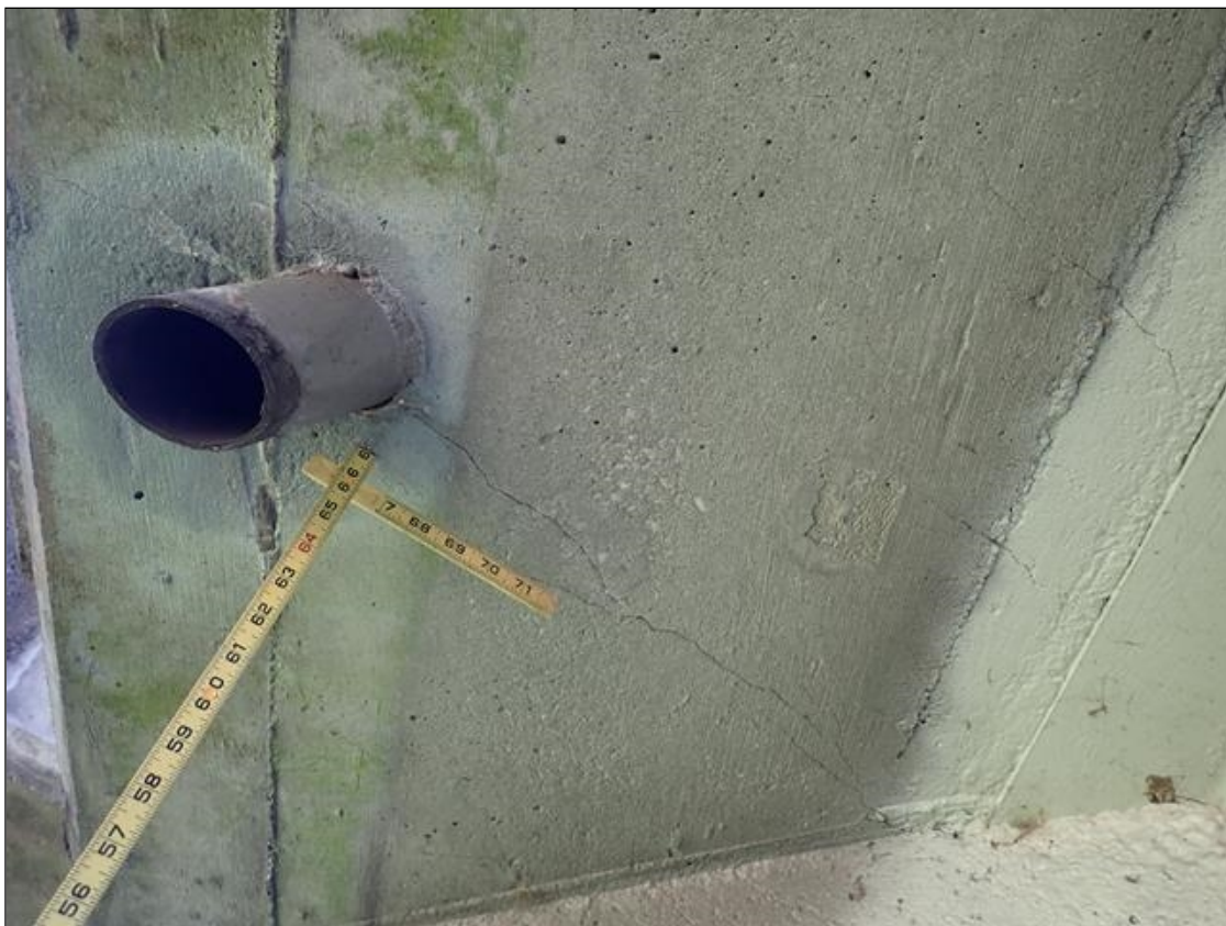
Span 1 Deck: UP TO 1/32 INCH WIDE TRANSVERSE CRACKS UNDER LEFT OVERHANG, SCATTERED.
