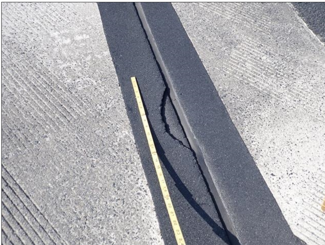
Span 1 End bent 1 Joint: span 1 side, in left travel lane near yellow line, spall/settlement (12 inch x 3 inch x 3/8 inch deep)
