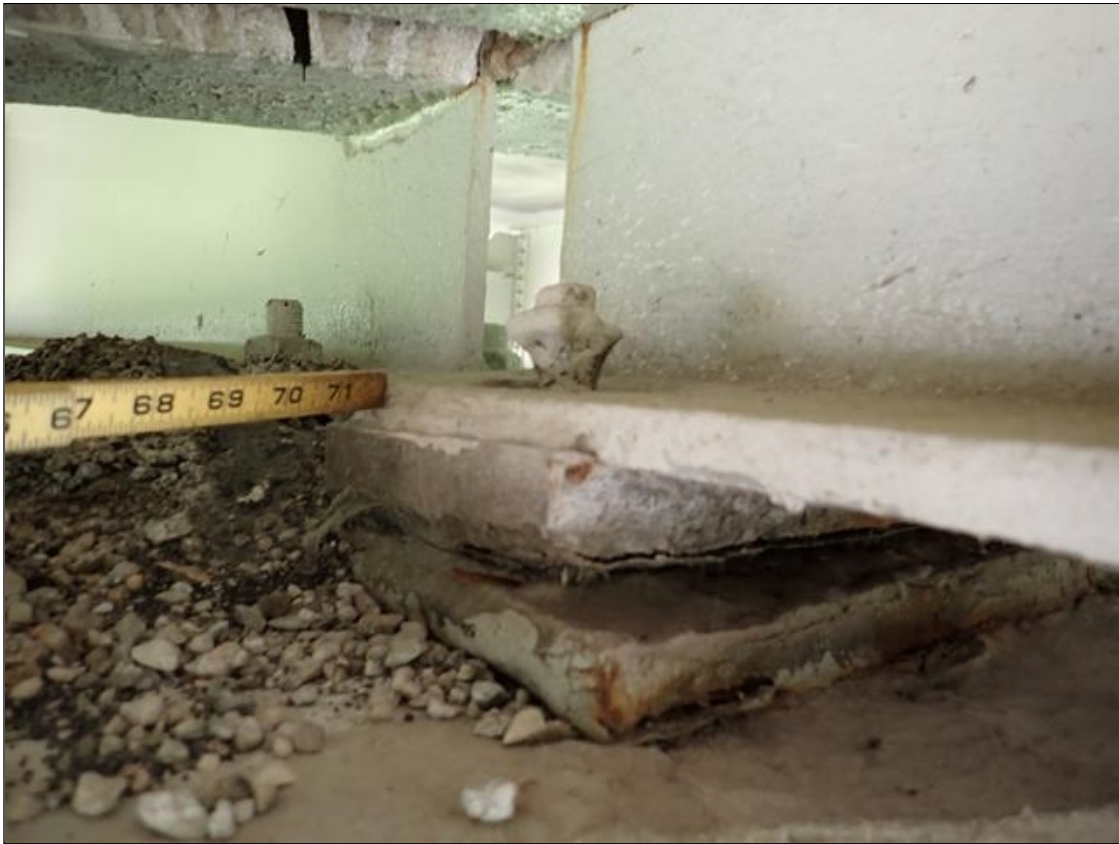
Span 6 Far Bearing 3: (PAR) LEFT ANCHOR BOLT HAS UP TO 80 PERCENT SECTION REMAINING AND ANCHOR BOLT NUT HAS UP TO 50 PERCENT SECTION REMAINING.
