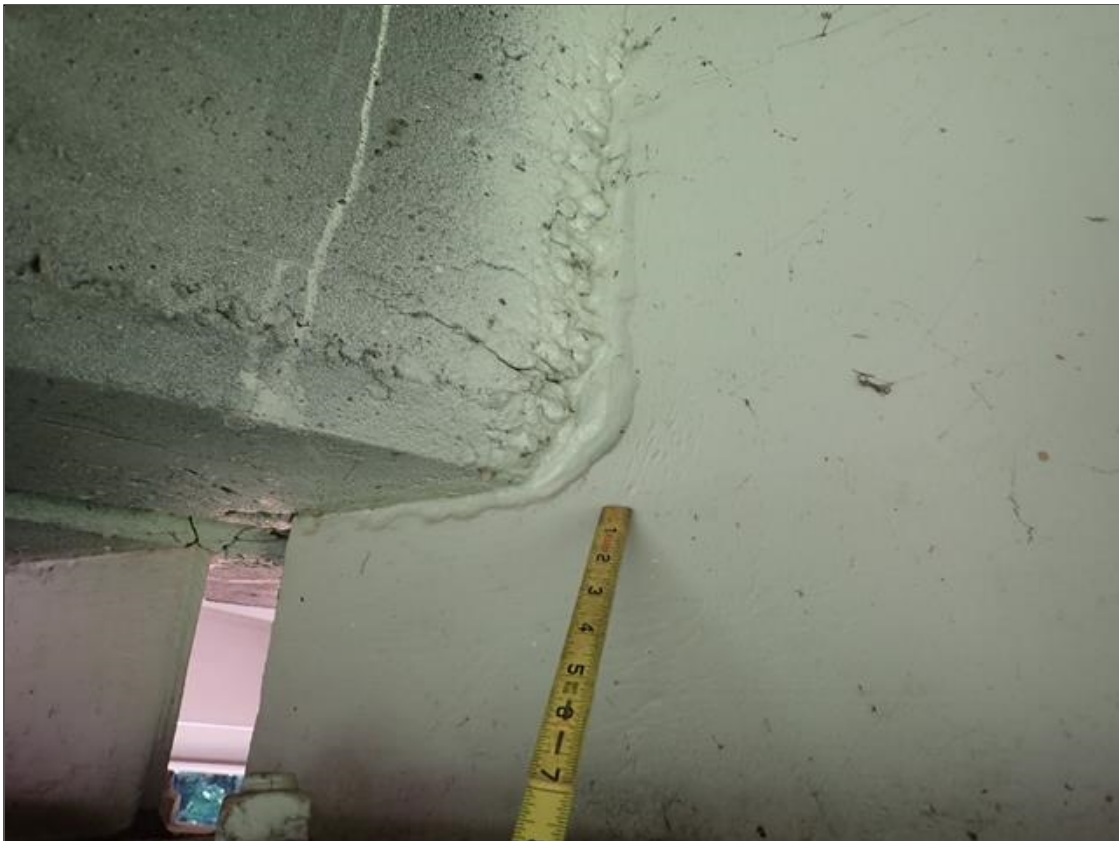
Span 3 Beam 2: (PAR) at bent 3, web adjacent to end diaphragm, painted over section loss (3/8 inch average remaining x 8 inch x 7 inch)
