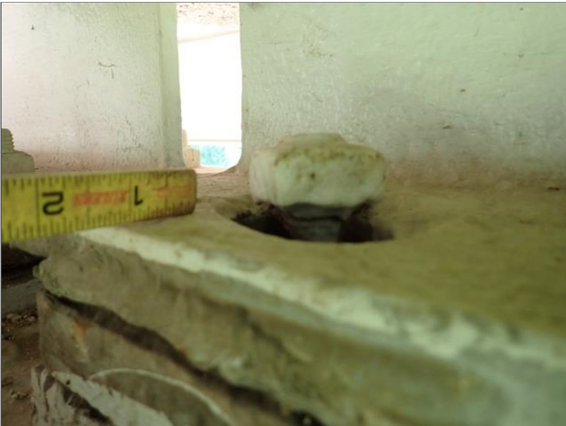
Span 3 Far Bearing 3: (PAR) ANCHOR BOLT NUT NOT CONNECTED COMPLETELY. SECTION LOSS WITH 70 PERCENT OF BOLT AND NUT REMAINING. HAS BEEN PAINTED.
