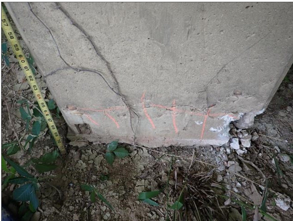
Bent 7 Pile 6: UP TO 3 INCHES HIGH OF THE STEEL PILE EXPOSED AT THE BOTTOM EXHIBITS SURFACE CORROSION WITH NO MEASUREABLE SECTION LOSS IN THE FLANGES AND WEB. CONCRETE REPAIR AT BASE OF PILE COVERS STEEL PILE; AT BASE, SOUTH FACE, DELAMINATION/SPALL (22 INCH X 6 INCH X 3 INCH DEEP)
