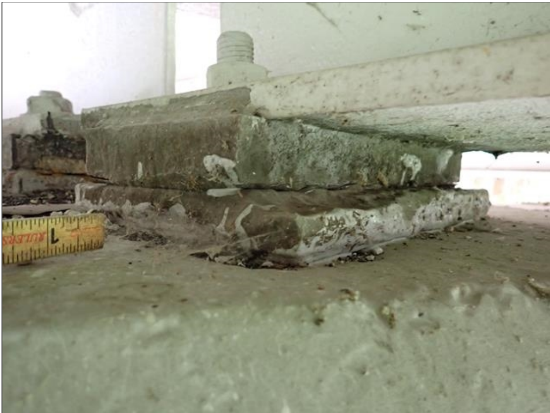
Span 7 Near Bearing 2: painted over section loss (approximately 85 percent remaining)
