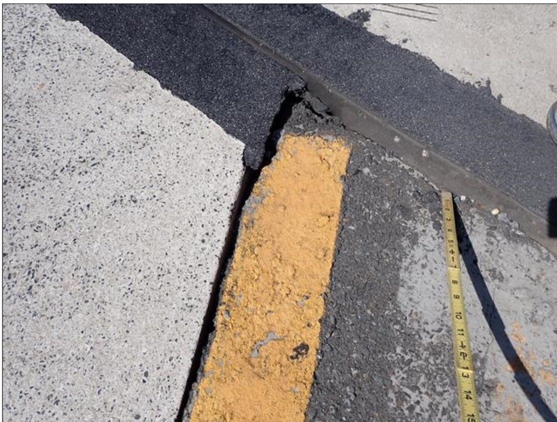
Approach 2: at west end adjacent to end bent 2 joint, settlement (12 inch x 16 inch x 1 inch deep)
