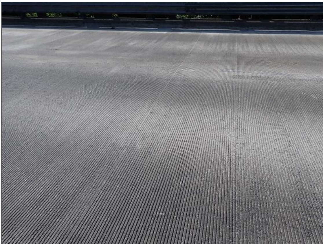
Span 1 Deck: throughout top of deck, wear with secure aggregate at random
