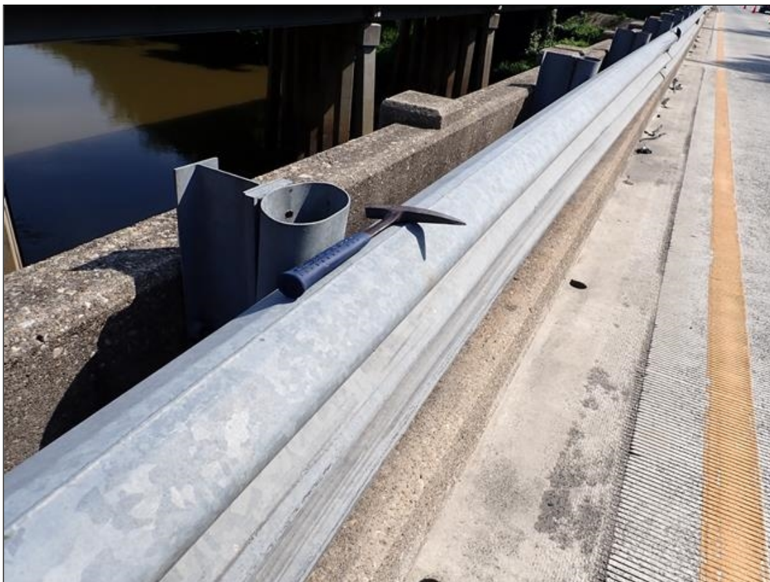
Span 5 Left Retrofit Bridge Rail: (PAR) starting at bent 4, impact damage (25 foot) with (3) partially crushed posts
