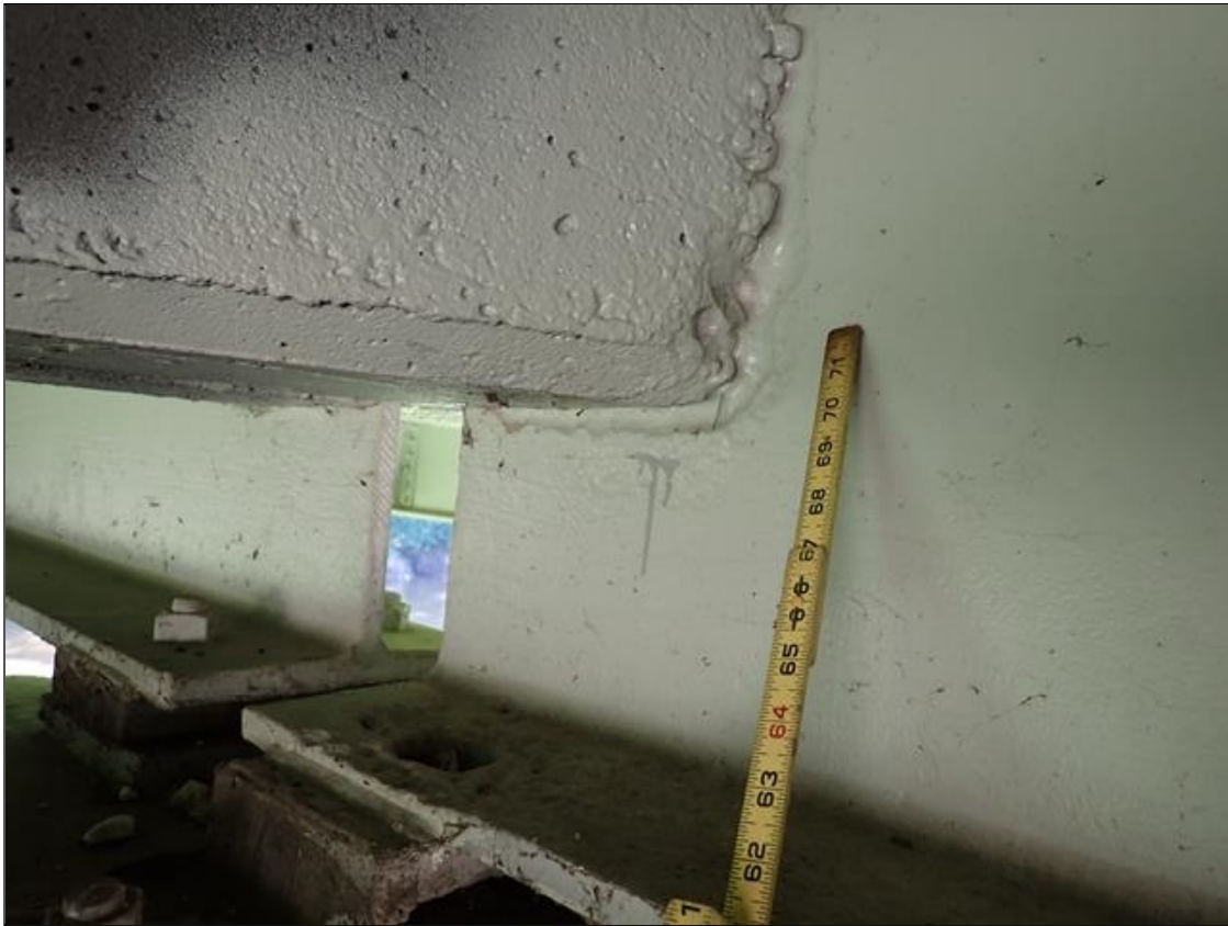
Span 1 Beam 3: (PAR) at bent 1, painted over section loss: web adjacent to end diaphragm (3/8 inch average remaining x 18 inch x 9 inch); bottom flange (0.65 inch average remaining x 8 inch)
