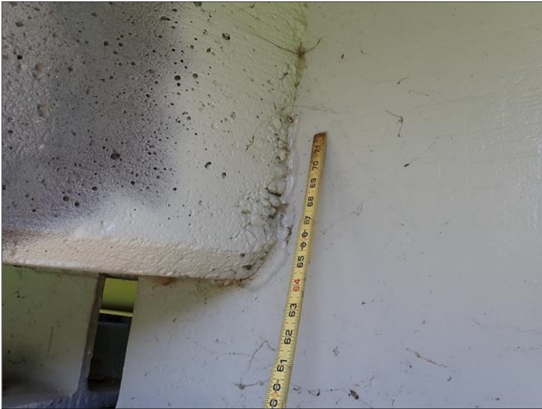
Span 2 Beam 4: (PAR) at bent 1, web adjacent to end diaphragm, painted over section loss (3/8 inch average remaining x 1 inch x 9 inch)
