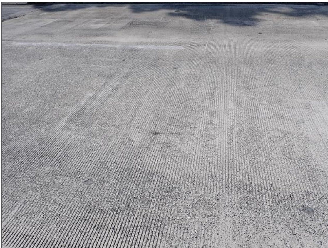
Approach 2: throughout slab, wear with secure aggregate at random
