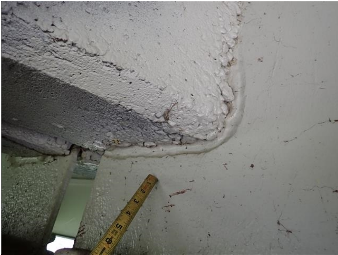
Span 7 Beam 3: (PAR) at bent 7, web adjacent to end diaphragm, painted over section loss (3/8 inch average remaining x 8 inch x 8 inch)
