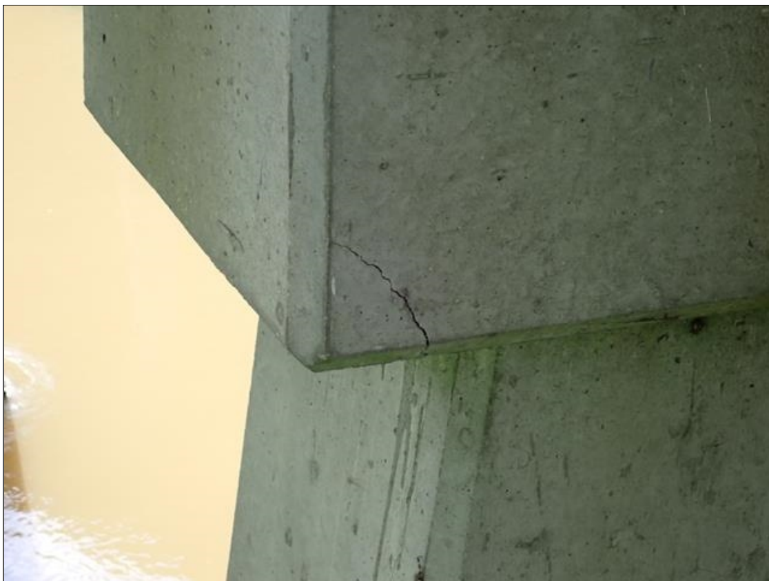
Bent 7 Cap 1: north face at east end, diagonal crack (1/16 inch x 6 inch)
