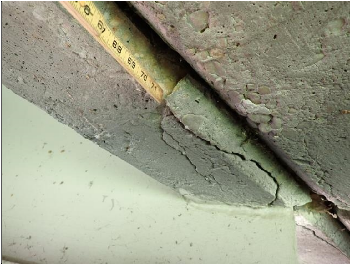
Span 3 Deck: 4 FEET LONG X 1 FOOT HIGH X 1.5 INCH DEEP FAILED PATCH IN BAY 1 DIAPHRAGM; ADJA TO BEAM 2, DELAMINATION (3 FOOT X 8 INCH) AT BENT 2.
