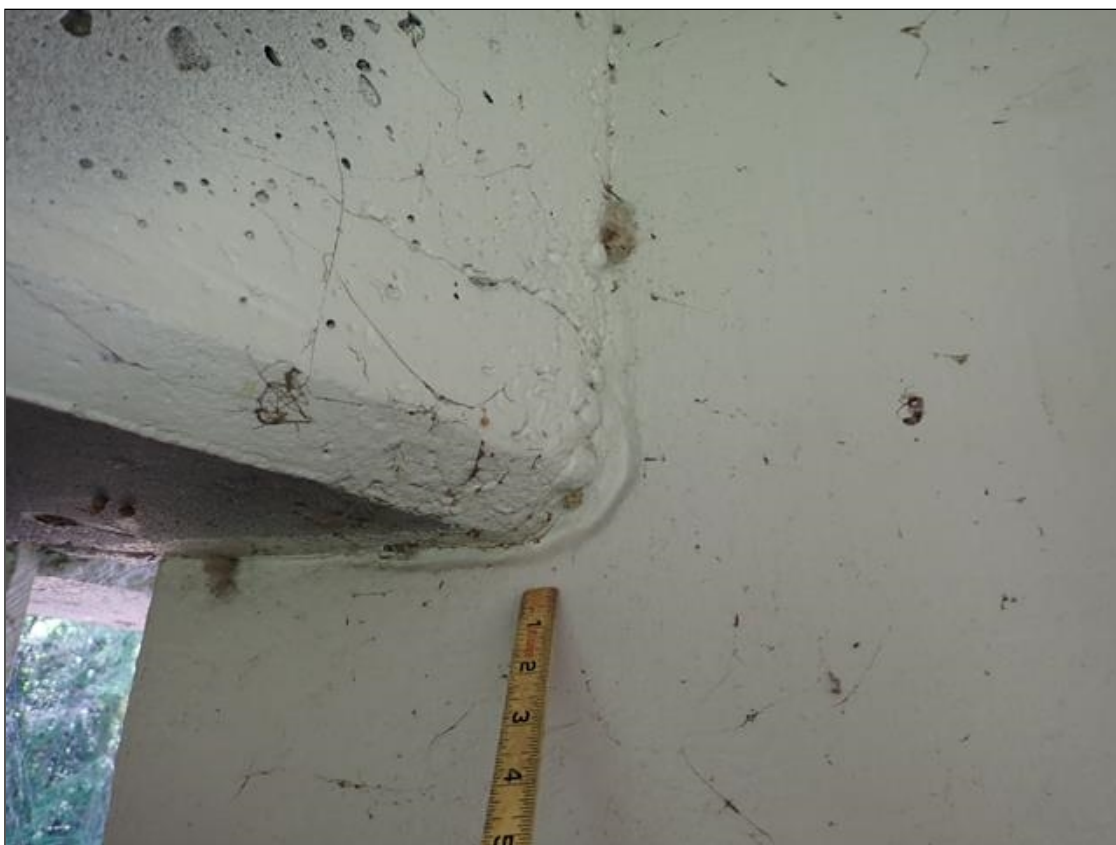
Span 3 Beam 4: (PAR) at bent 3, web adjacent to end diaphragm, painted over section loss (3/8 inch average remaining x 8 inch x 7 inch)
