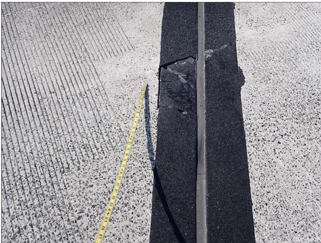
Span 3 Bent 2 Joint: span 3 side, at centerline, area of broken/cracked header with settlement (14 inch x 8 inch x 1/2 inch deep)
