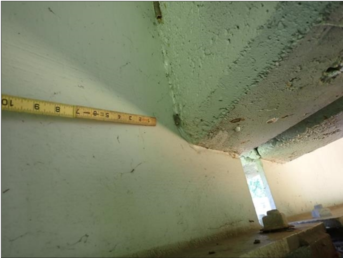
Span 3 Beam 1: at bent 3, web adjacent to end diaphragm, painted over section loss (1/2 inch average remaining x 7 inch x 1 inch)
