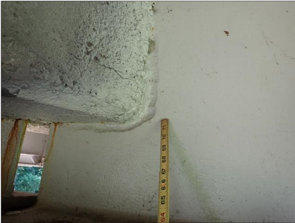
Span 4 Beam 2: (PAR) at bent 4, web adjacent to end diaphragm, painted over section loss (3/8 inch average remaining x 8 inch x 8 inch) with corrosion reactivating
