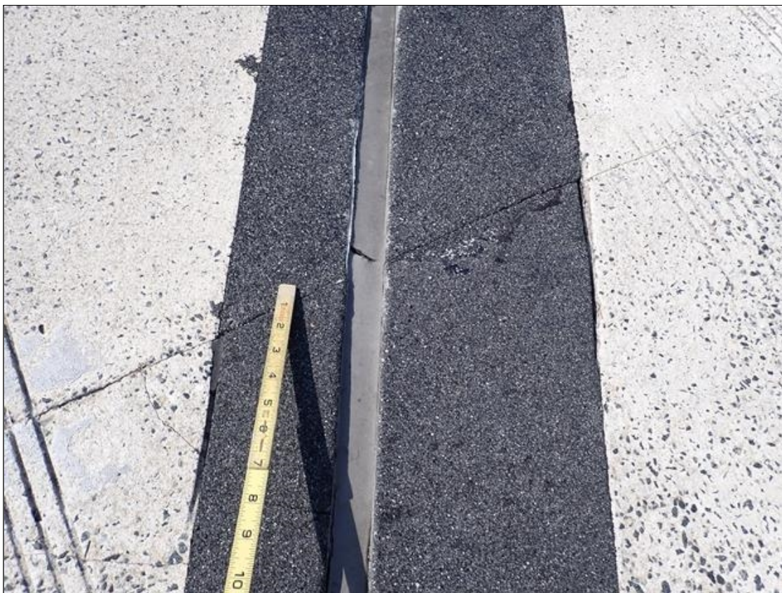
Span 5 Bent 4 Joint: at centerline of roadway, tear (1 inch long)
