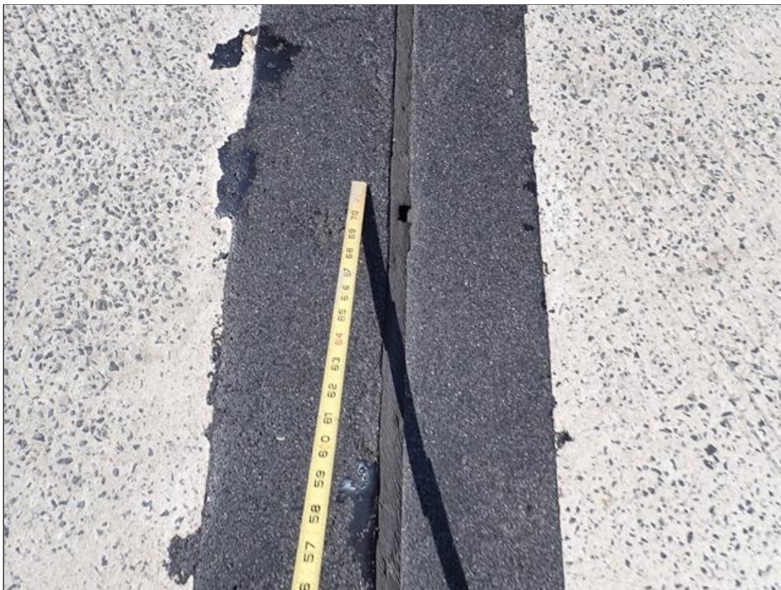
Span 8 End bent 2 Joint: in right travel lane, (2) area of missing seal (up to 1 inch diameter)
