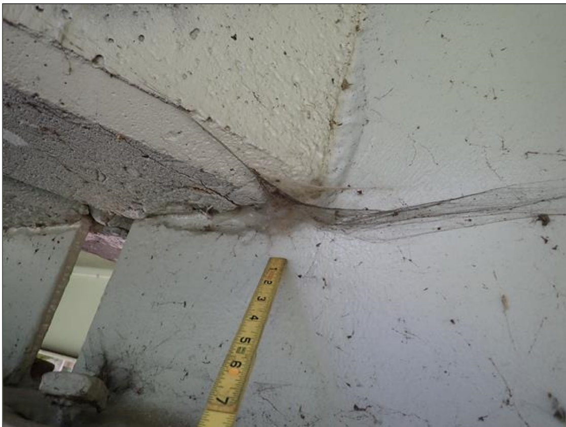
Span 8 Beam 4: (PAR) at bent 7, web adjacent to end diaphragm, painted over section loss (3/8 inch average remaining x 7 inch x 8 inch)
