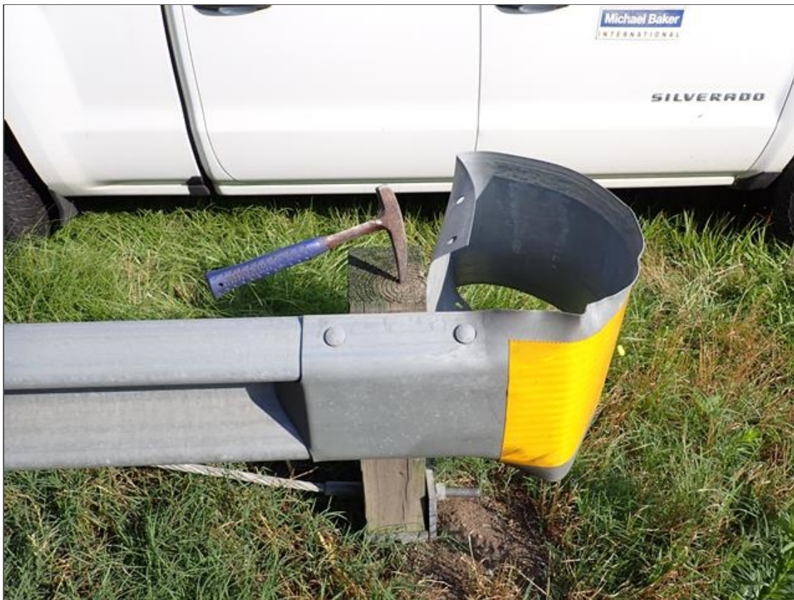
(PAR) northwest guardrail termination, impact damage
