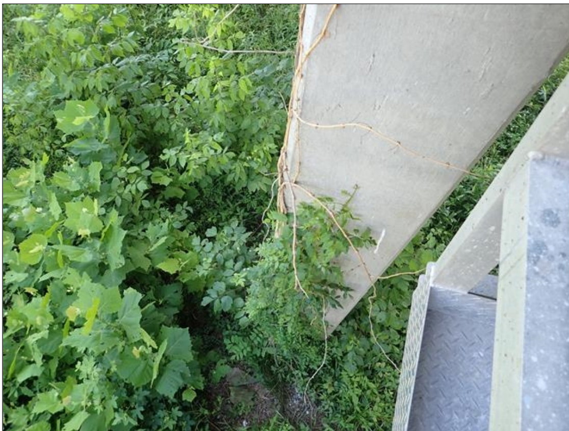
Bent 1 Pile 1: along pile, vegetation growth
