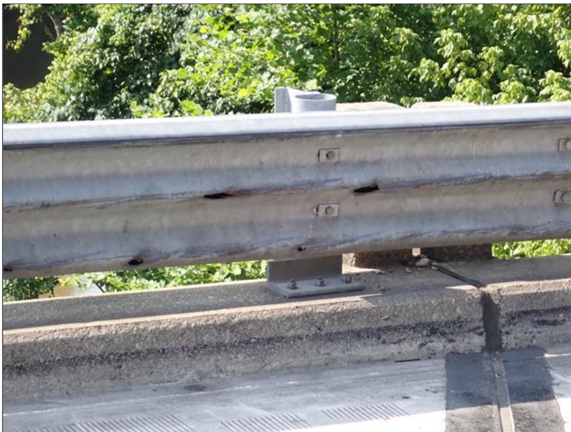
Span 3 Right Retrofit Bridge Rail: (PAR) IMPACT DAMAGE WITH SCRAPE MARKS AND THROUGH HOLES UP TO 4 INCH X 2 INCH IN RETROFIT RAIL AT SCATTERED LOCATIONS
