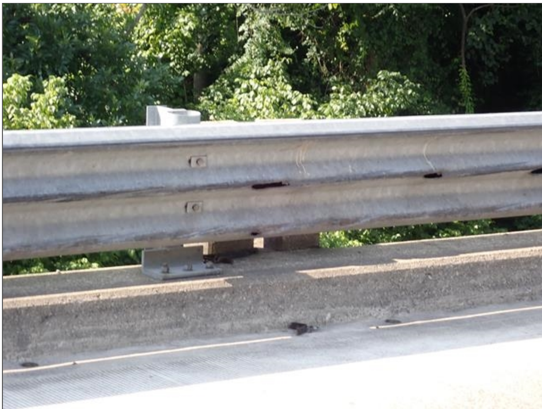
Span 2 Right Retrofit Bridge Rail: (PAR) IMPACT DAMAGE WITH SCRAPE MARKS AND THROUGH HOLES UP TO 3 INCH X 2 INCH IN RETROFIT RAIL AT SCATTERED LOCATIONS
