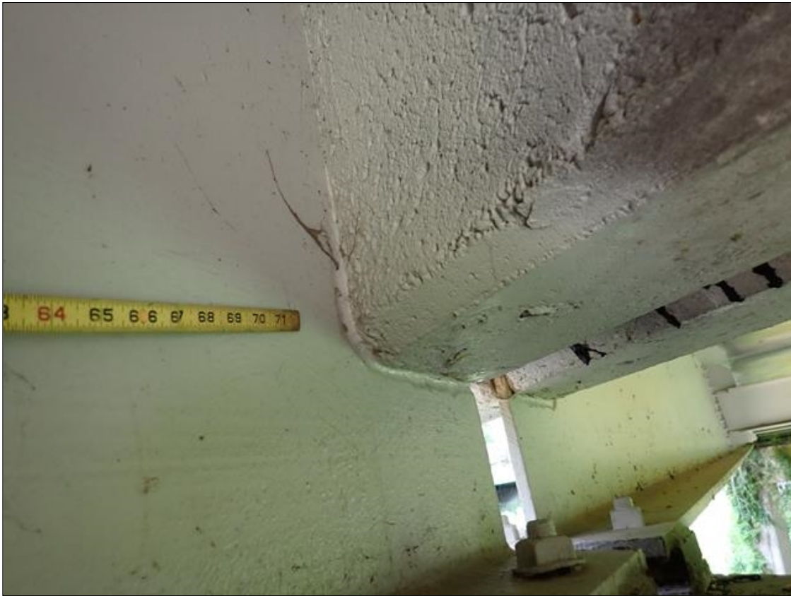
Span 6 Beam 1: (PAR) at bent 6, web adjacent to end diaphragm, painted over section loss (3/8 inch average remaining x 8 inch x 4 inch) with corrosion reactivating
