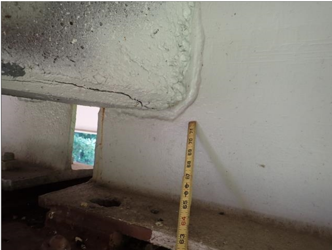
Span 4 Beam 3: (PAR) at bent 4, web adjacent to end diaphragm, painted over section loss (3/8 inch average remaining x 8 inch x 8 inch) with corrosion reactivating
