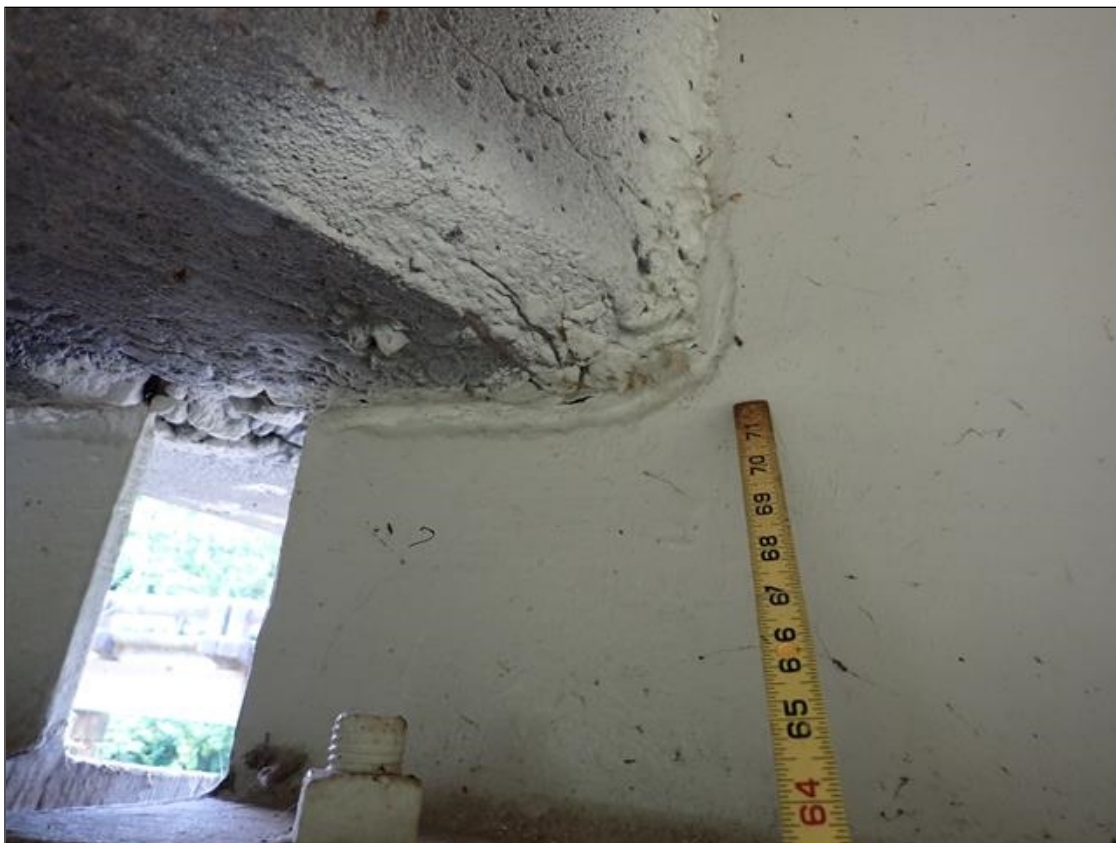
Span 6 Beam 1: (PAR) at bent 5, web adjacent to end diaphragm, painted over section loss (3/8 inch average remaining x 8 inch x 8 inch)
