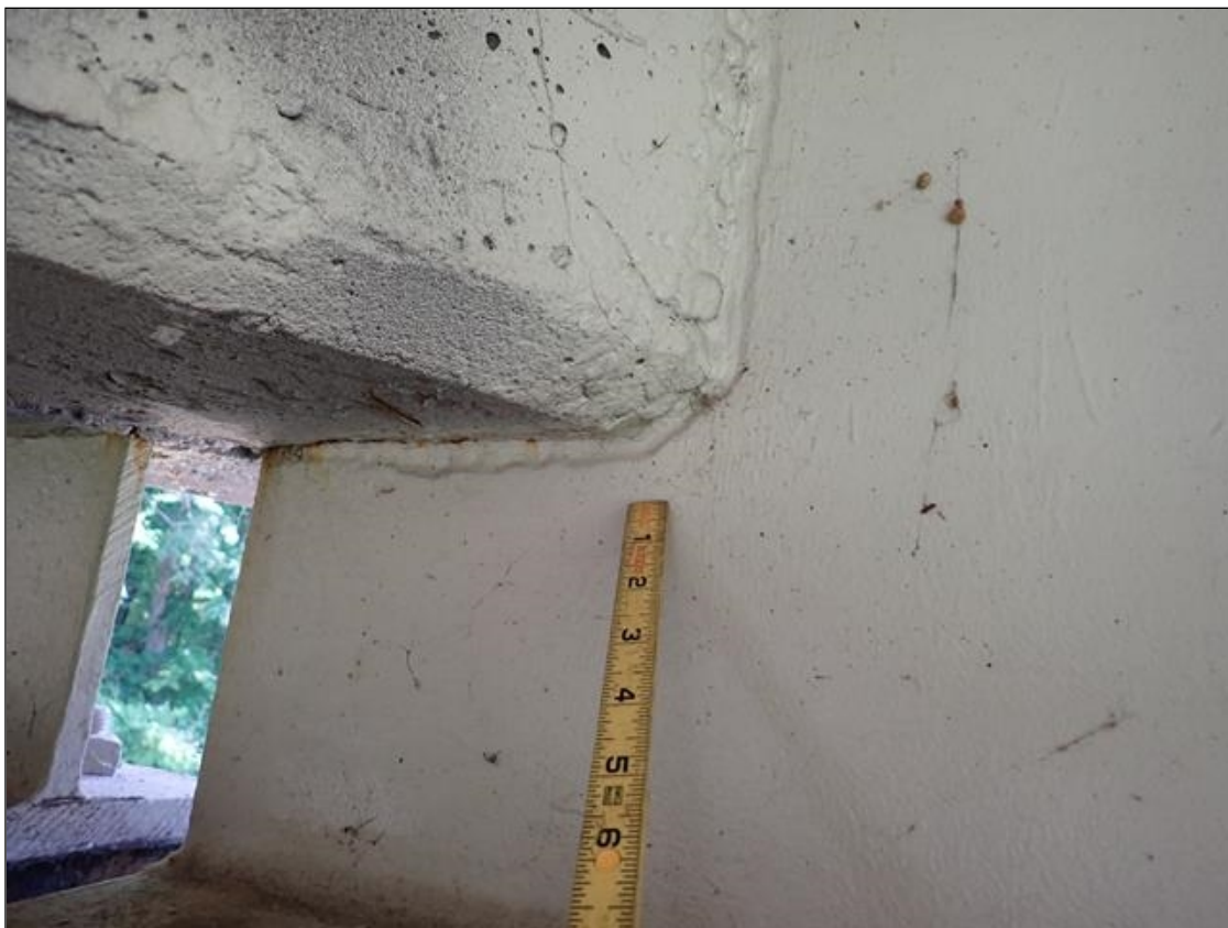
Span 4 Beam 4: (PAR) at bent 4, web adjacent to end diaphragm, painted over section loss (3/8 inch average remaining x 8 inch x 8 inch)
