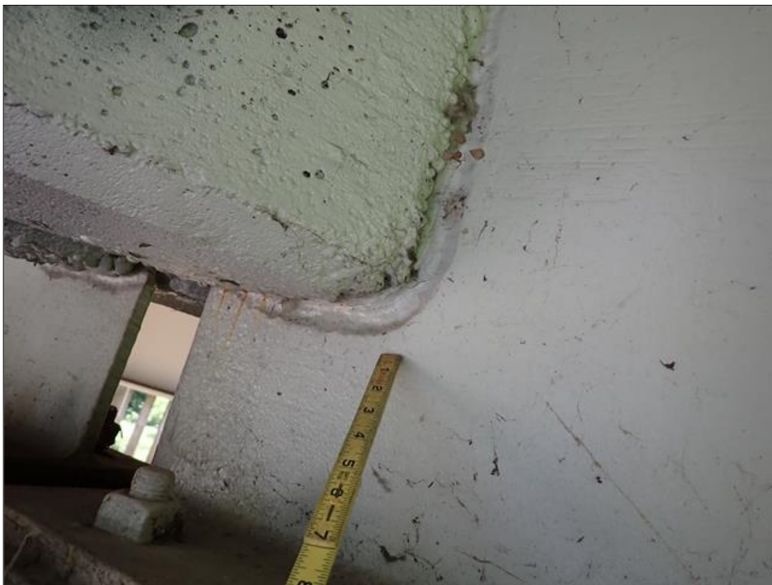
Span 7 Beam 4: (PAR) at bent 6, web adjacent to end diaphragm, painted over section loss (3/8 inch average remaining x 7 inch x 12 inch) with corrosion reactivating
