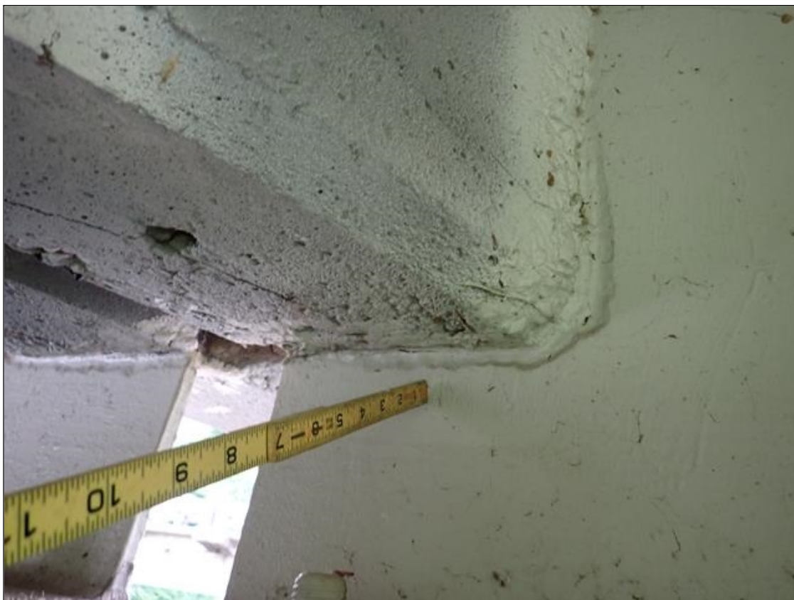
Span 7 Beam 1: (PAR) at bent 6, web adjacent to end diaphragm, painted over section loss (3/8 inch average remaining x 7 inch x 14 inch) with corrosion reactivating
