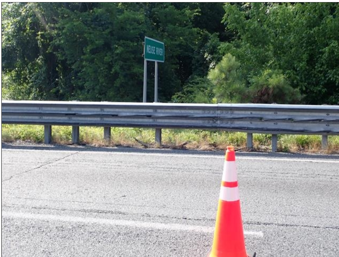
(PAR) southeast guardrail, starting at bridge, impact damage (30 foot)
