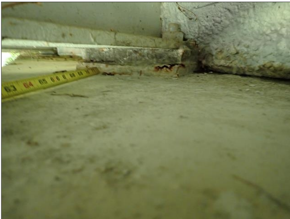
Span 1 Near Bearing 2: painted over section loss (approximately 80 percent remaining) with corrosion reactivating
