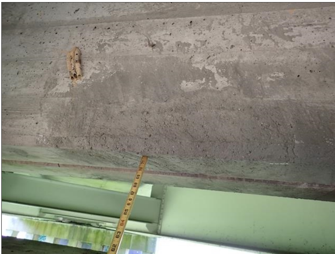
Span 3 Deck: BAY 2, END DIAPHRAGM, AT BENT 2, 2 FEET LONG X 1 FOOT HIGH SOUND PATCH.
