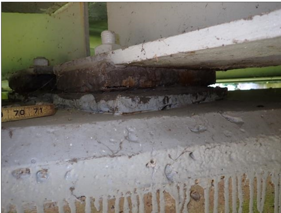
Span 3 Near Bearing 3: painted over section loss (less than 1/16 inch loss) with corrosion reactivating
