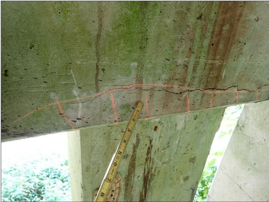
Bent 7 Cap 1: 3 FEET WIDE X 6 INCHES HIGH DELAMINATION WITH A 3 FEET LONG HORIZONTAL CRACK UP TO 1/16 INCH WIDE BOTTOM OF NORTH FACE, OVER PILE 3.
