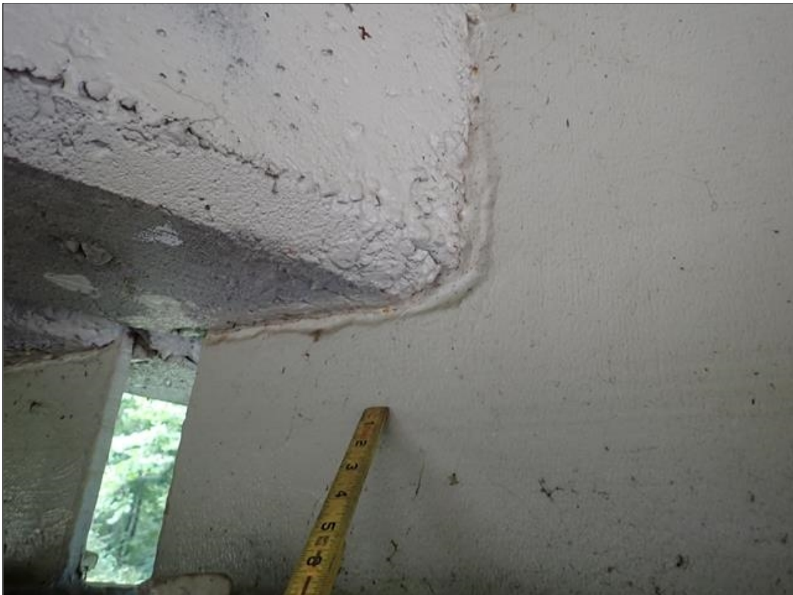
Span 7 Beam 4: (PAR) at bent 7, web adjacent to end diaphragm, painted over section loss (3/8 inch average remaining x 7 inch x 5 inch) with corrosion reactivating
