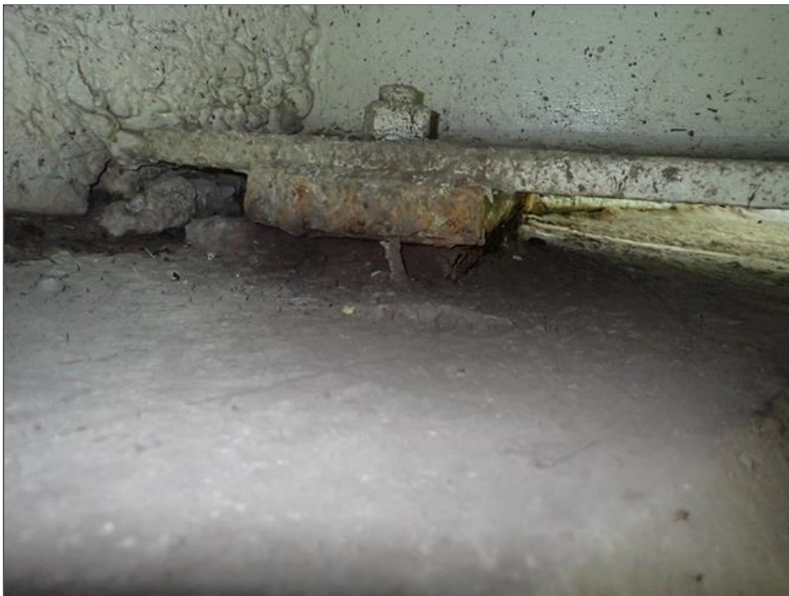
Span 8 Far Bearing 4: corrosion with section loss (approximately 80 percent remaining)
