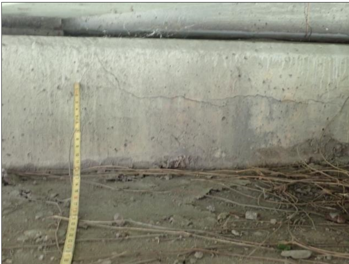
End Bent 2 Cap 1: UP TO 3 FEET LONG X 1/16 INCH WIDE HORIZONTAL CRACK, BELOW BEAM 2. TYPICAL AT BEAM 3.
