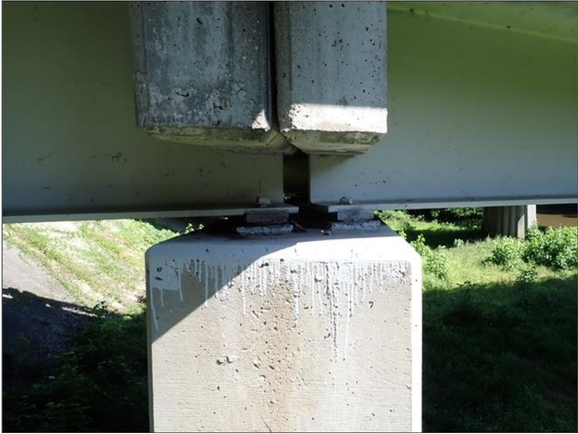
beams over bent
