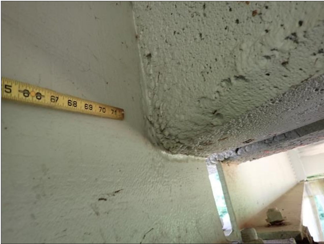
Span 6 Beam 4: at bent 5, web adjacent to end diaphragm, painted over section loss (9/16 inch average remaining x 8 inch x 8 inch)
