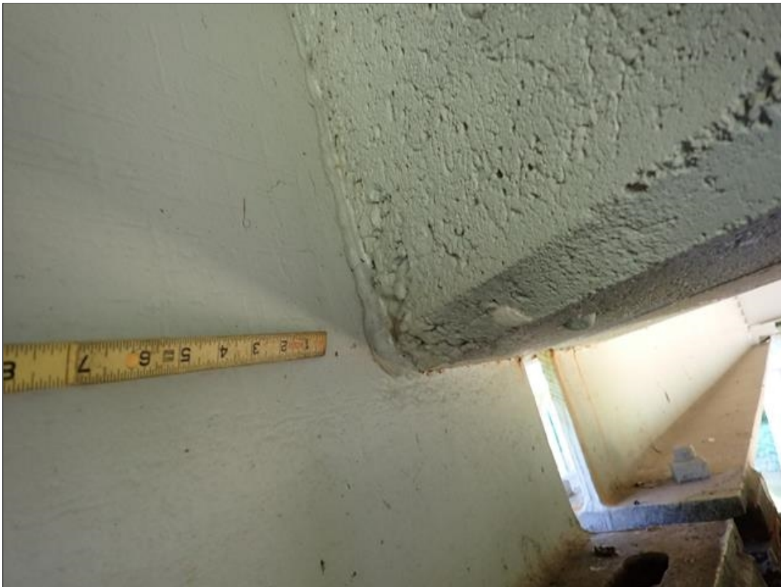
Span 4 Beam 1: (PAR) at bent 4, web adjacent to end diaphragm, painted over section loss (3/8 inch average remaining x 8 inch x 1 inch)
