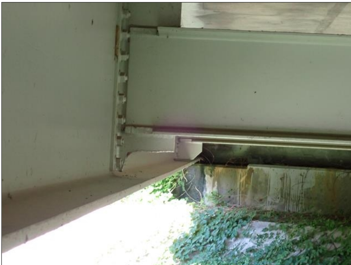
Span 1 Beam 4 : 2 INCHES HIGH OF INTERMEDIATE STIFFENER IS CUT OUT AT BOTTOM AT BOTH LOCATIONS. PAR IS NOT ISSUED AS IT APPEARS TO BE FROM PREVIOUS BRIDGE REPAIR.
