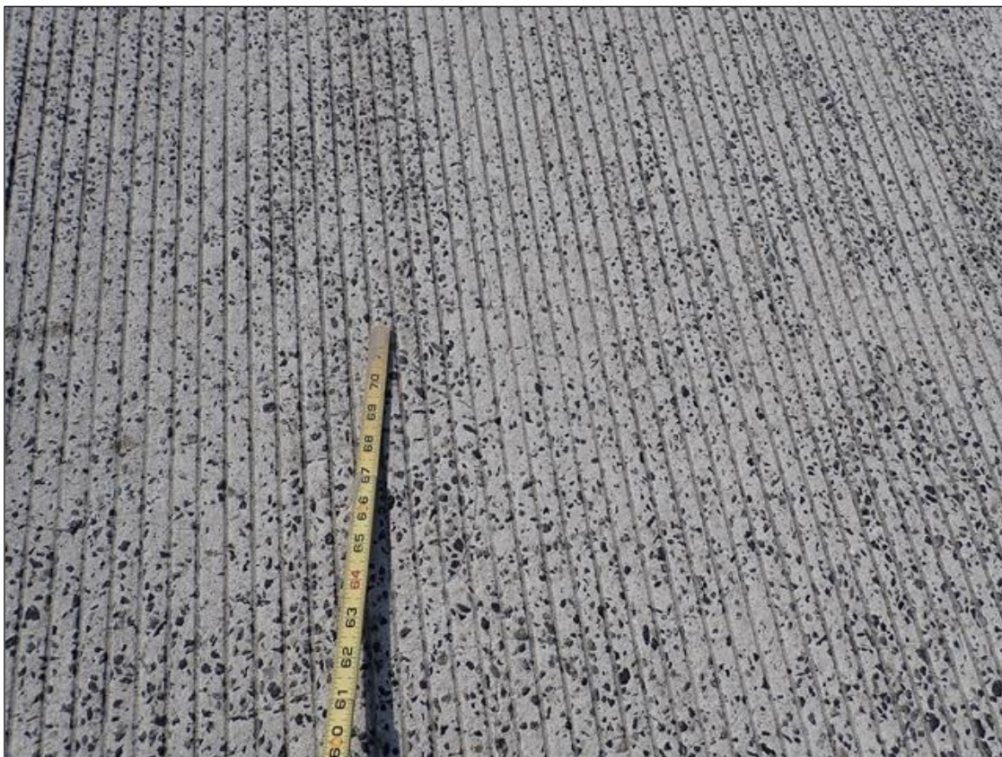
Span 4 Deck: throughout top of deck, areas of map cracks (hairline) at random
