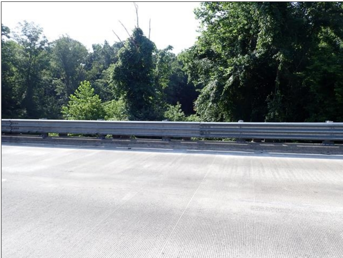
Span 1 Right Retrofit Bridge Rail: (PAR) IMPACT DAMAGE WITH SCRAPE MARKS AND THROUGH HOLES UP TO 3 INCH X 2 INCH IN RETROFIT RAIL AT SCATTERED LOCATIONS
