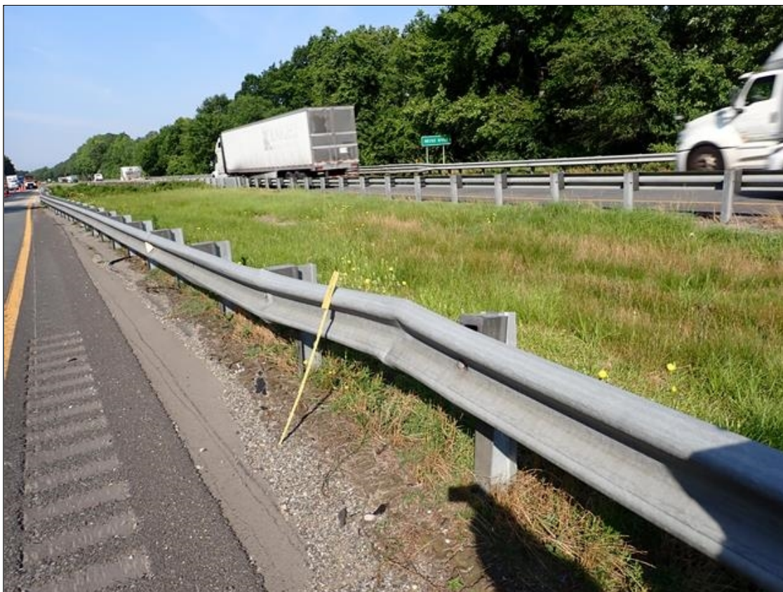
(PAR) northwest guardrail, approximately 60 foot from bridge, impact damage (10 foot)
