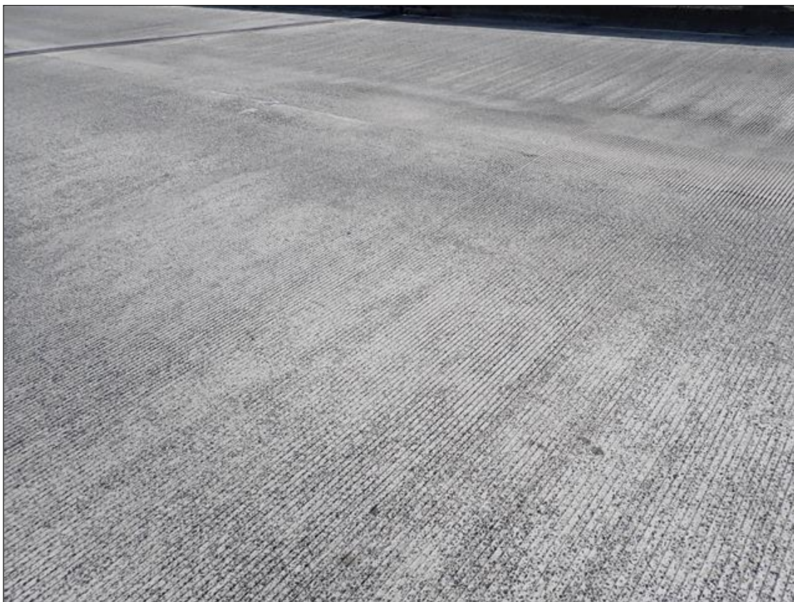
Span 4 Deck: throughout top of deck, wear with secure aggregate at random
