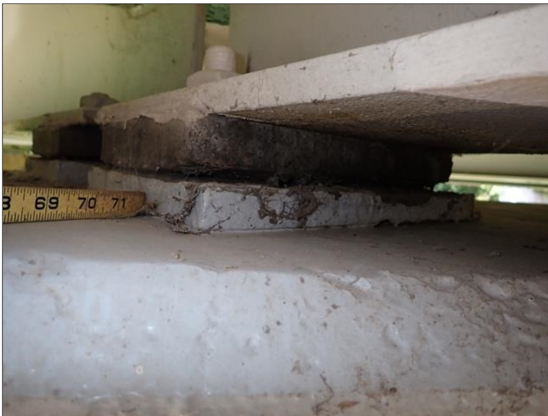
Span 4 Near Bearing 3: painted over section loss (approximately 80 percent remaining)
